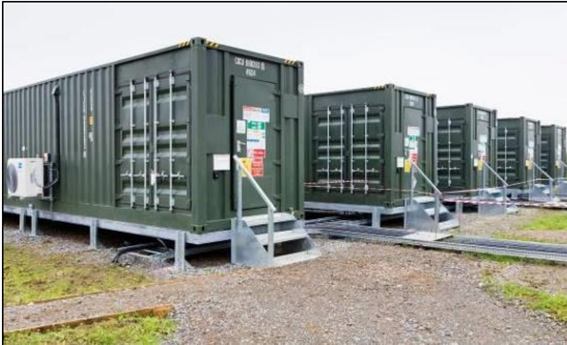
Photograph 1.2: Example of BESS located in storage containers
