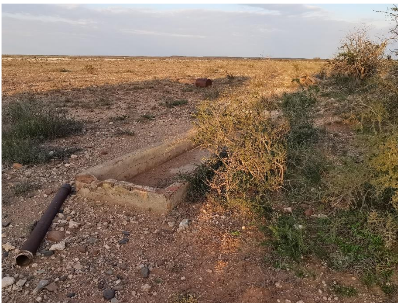
Figure 13: Water crib for livestock.
