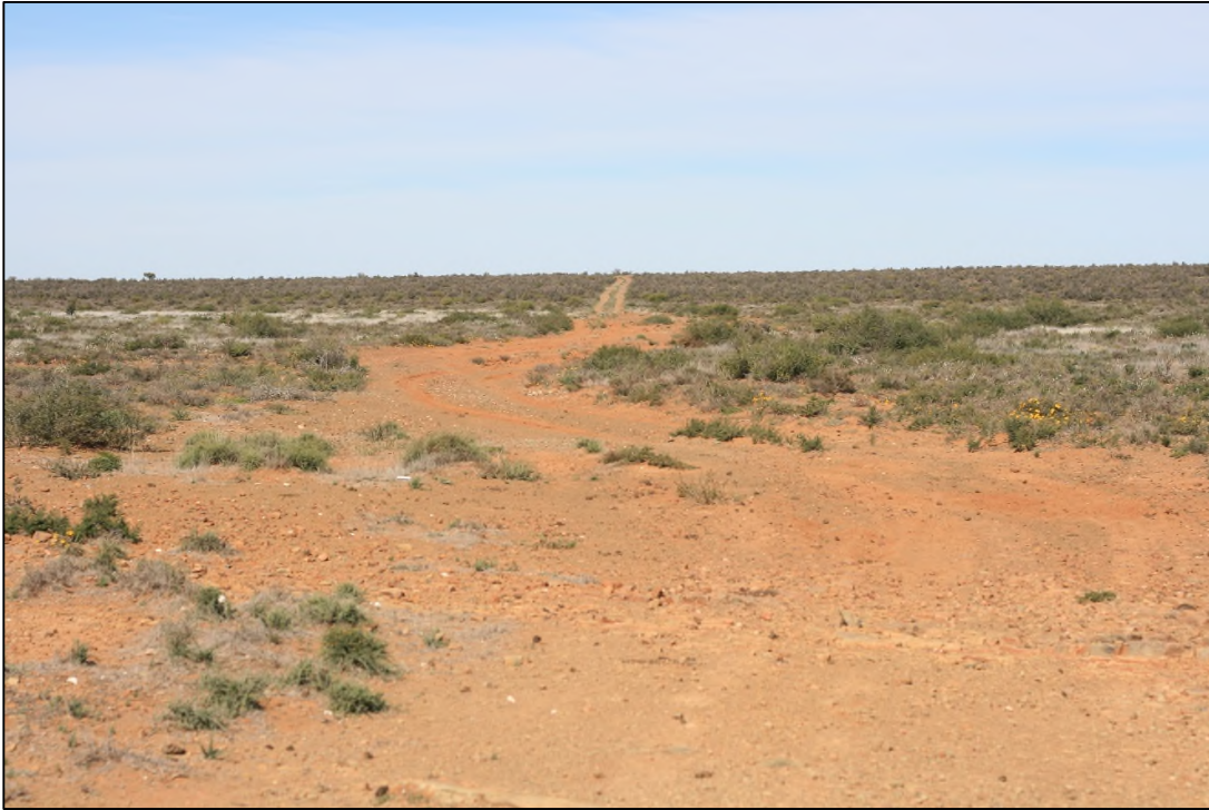
Photo 2-6 Erosion observed on a typical sand road
