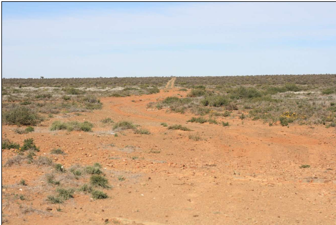
Photo 2-6 Erosion observed on a typical sand road
