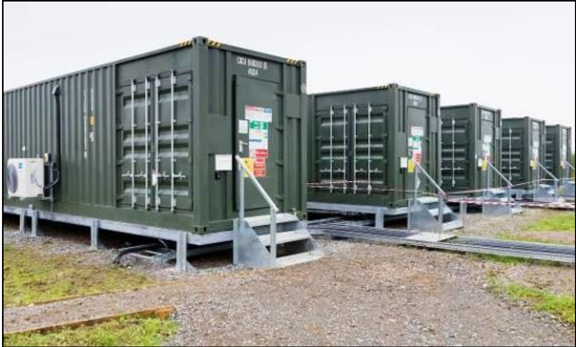
Photograph 1.2: Example of BESS located in storage containers
