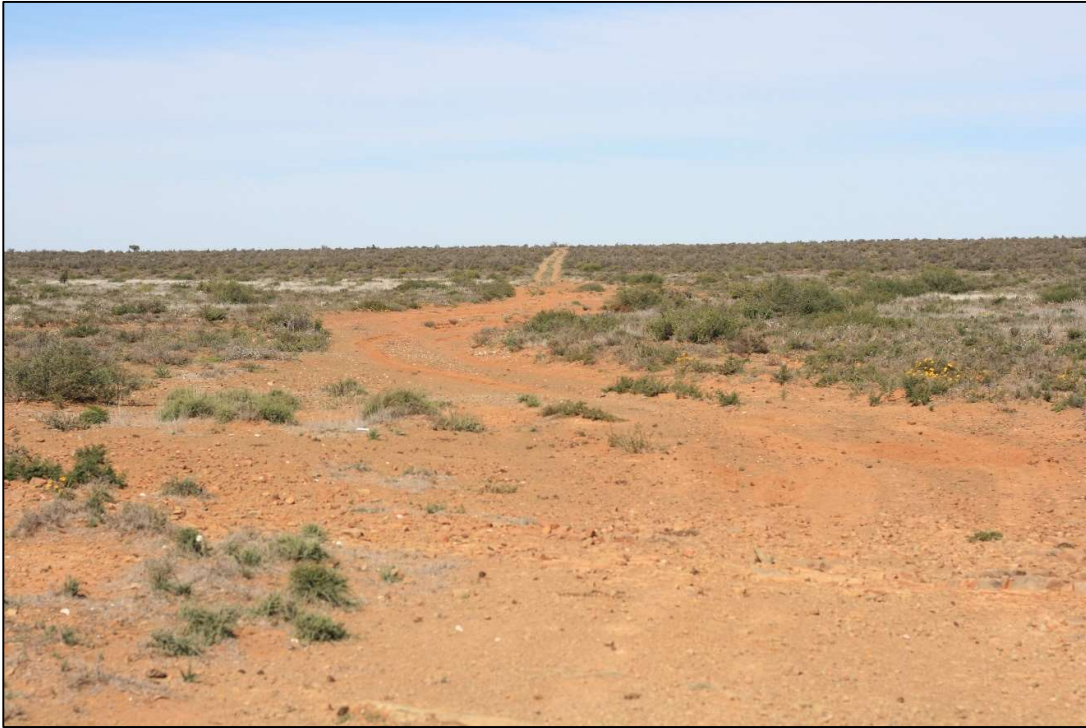
Photo 2-6 Erosion observed on a typical sand road
