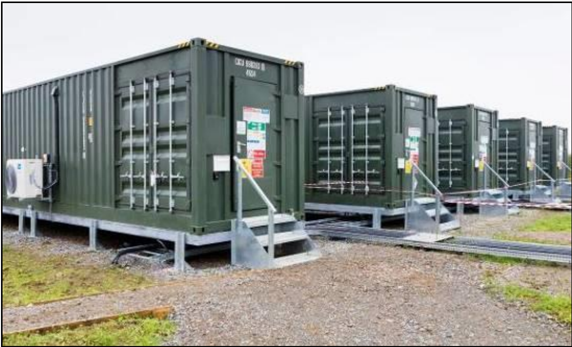
Photograph 1.2: Example of BESS located in storage containers
