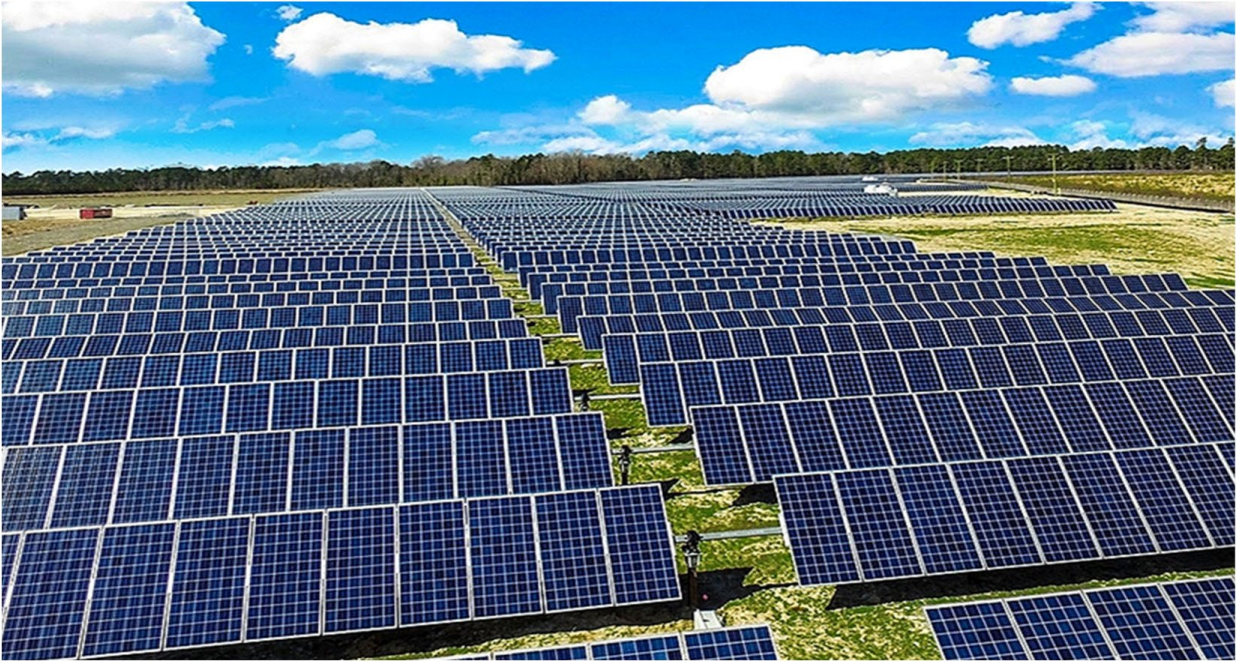
Figure 2.1: Typical example of solar PV array
