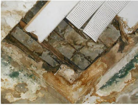
Fig.1 Image showing severe spalling(deterioration) to the existing suspended concrete slab.
