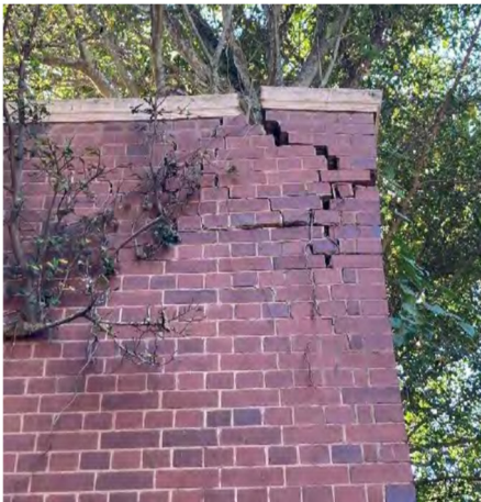
Fig.3 Image showing severe structural damage to the existing parapet wall.
