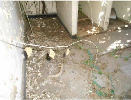
Fig.2 Image showing severe settlement of the existing surface bed slab in the ablutions.
