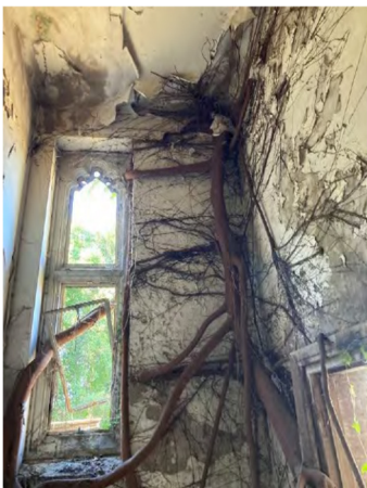
Fig.4 Image showing severe vegetation growth on the inside of the Chapel.
