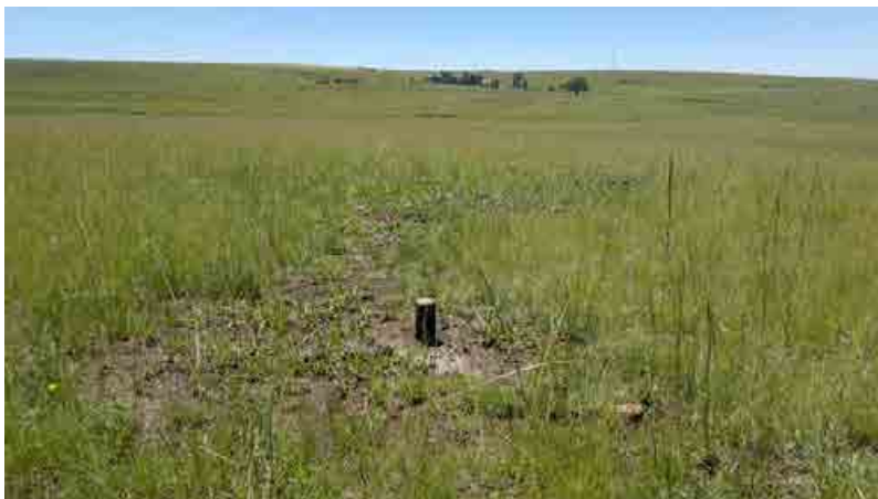
FIGURE 4-14: COMPLETED EXPLORATION BOREHOLE (STAND PIPE STILL TO BE CUT BELOW GROUND LEVEL)
