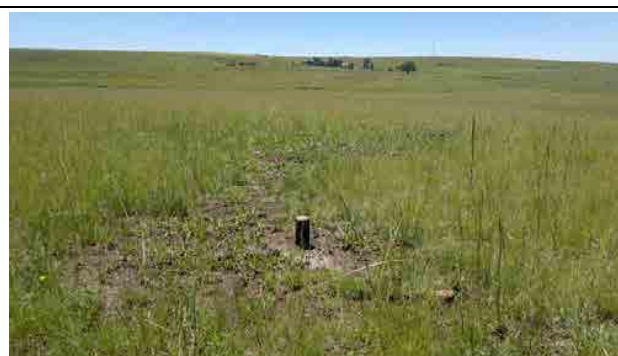
Figure 7: Completed exploration borehole (stand pipe still to be cut below ground level)
