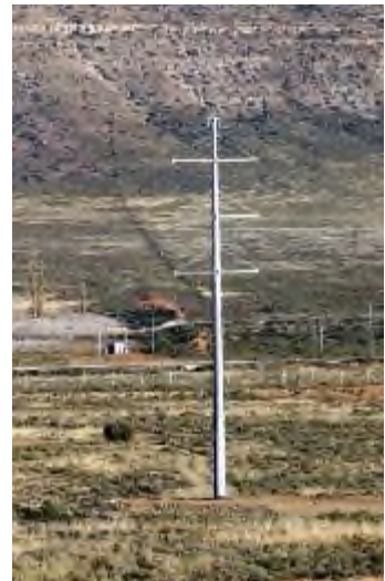
Plate 3, Eskom 220kV Monopole.
