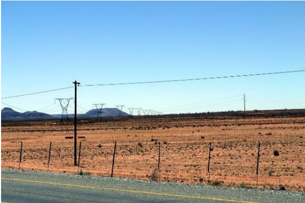
Plate 8, Aggeneis to Aries 400kV power line approaching the N14 from the direction of the proposed solar PV project. Power Line Corridor Alternative 1 is centred on this existing power line.
