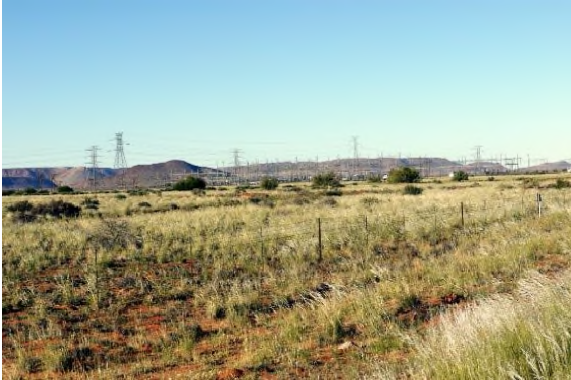
Plate 1, Existing Aggeneis Main Transformer Substation (MTS).
