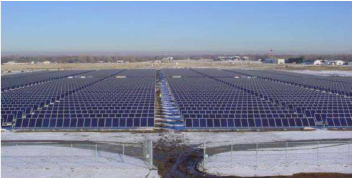
Plate 14 - PV array viewed from above. Note the array rows are read as one and have a similar impact as the roof of a large industrial building.
