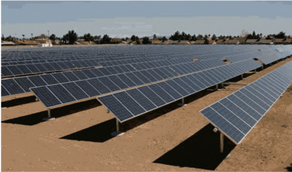
Plate 1. Fixed mounted PV system. Each unit is fixed in place orientated towards the sun's mid-day position. With a single-axis system each row would be placed in a north-south direction and the panels would be moving to follow the sun's position from sunrise to sunset.
