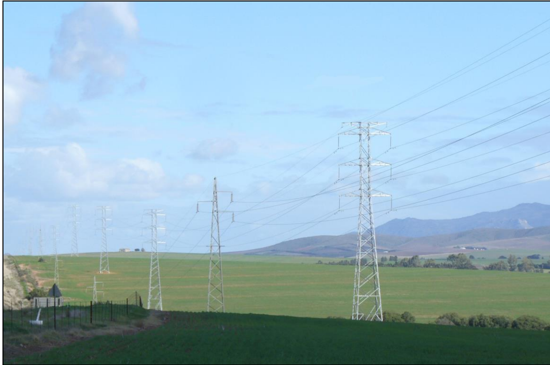
Figure 9: Examples of 132kV overhead power lines.
