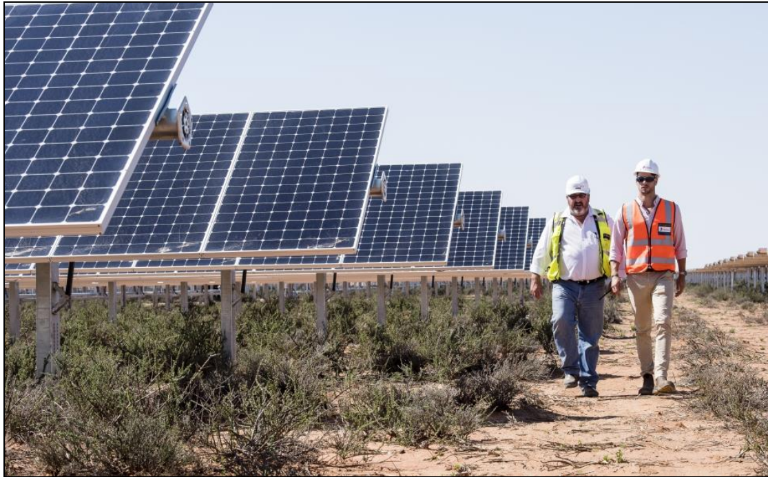
Figure 2: Photovoltaic (PV) solar panels. ( SunPower Solar Power Plant – Prieska ).
