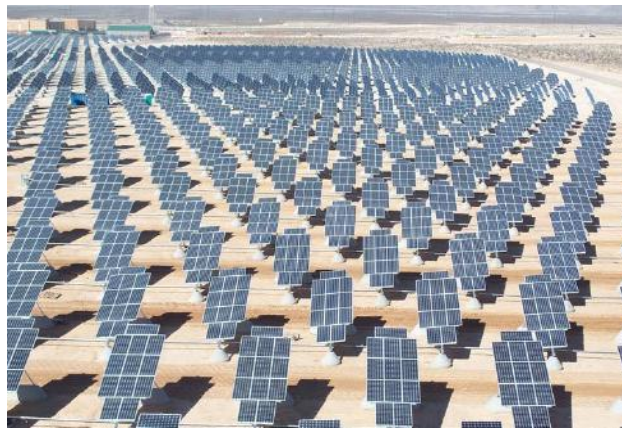
Figure 1: Photovolatic (PV) solar farm showing typical arrangement of photovoltaic panels.
