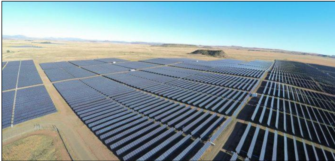
Figure 3: Aerial view of PV arrays. ( Scatec Solar South Africa ).
