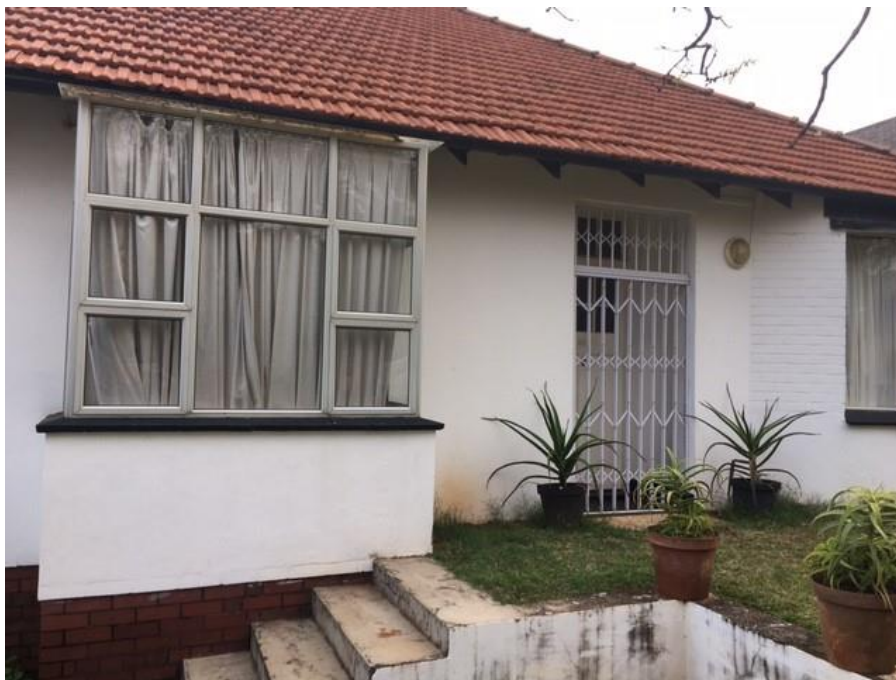
Photo 8 – Main entry to house Showing shocking hap hazard roof additions
