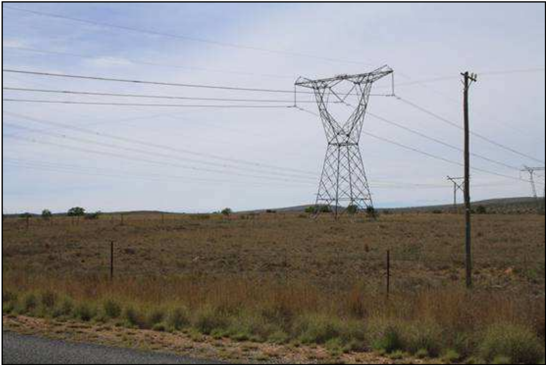
Figure 4: Transmission line infrastructure (Delphi-Poseidon and Hydro-Poseidon) crossing the R63 north-west of the proposed development area.
