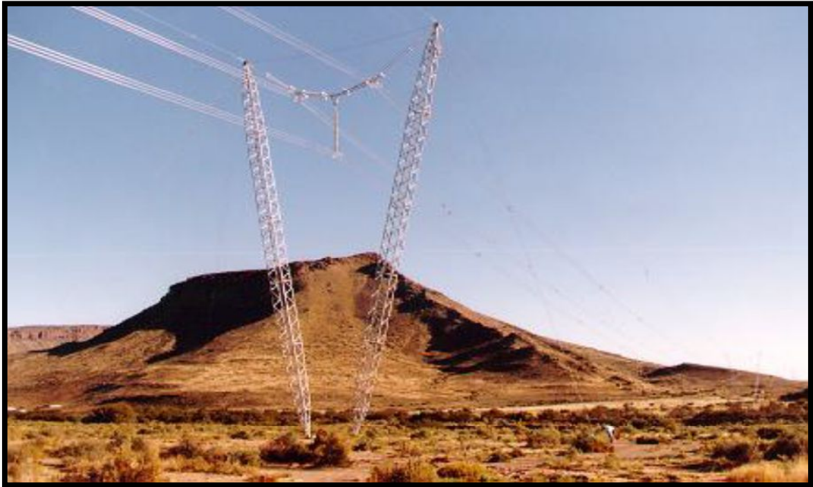
Figure 8: Guyed V structure
