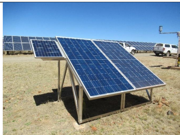
B: Soiling station installed to monitor and determine operational efficiencies in Lesedi south solar field.
