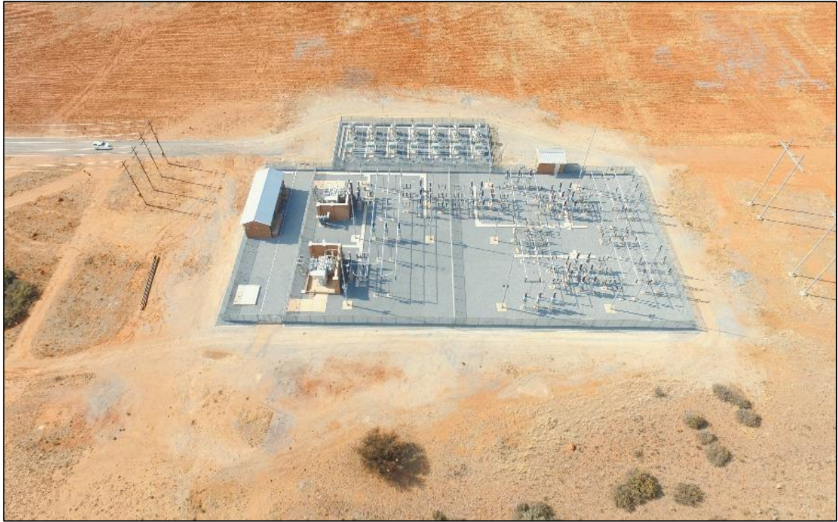
Figure 7: Substation, capacitor banks and grid connection
