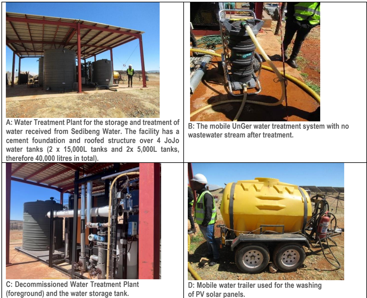
Figure 19: Water Treatment Plant
