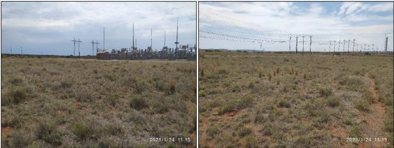
Figure 38: Open grassy vegetation around the substation (Vegetation Review, 2023)
