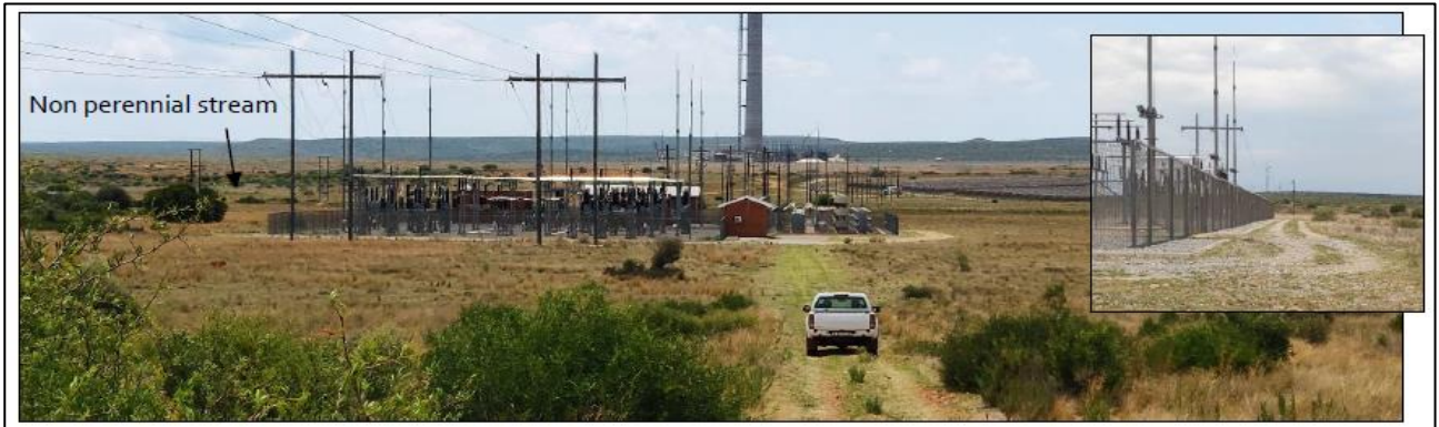
Figure 36: View of the substation, looking northwards, in a grass dominated landscape (Vegetation Review, 2023)
