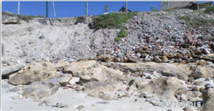
Figure 2.: Eroding harbour embankment
