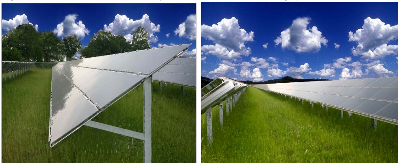
Figure 3 Lateral views of PV arrays mounted on fixed mounting systems
