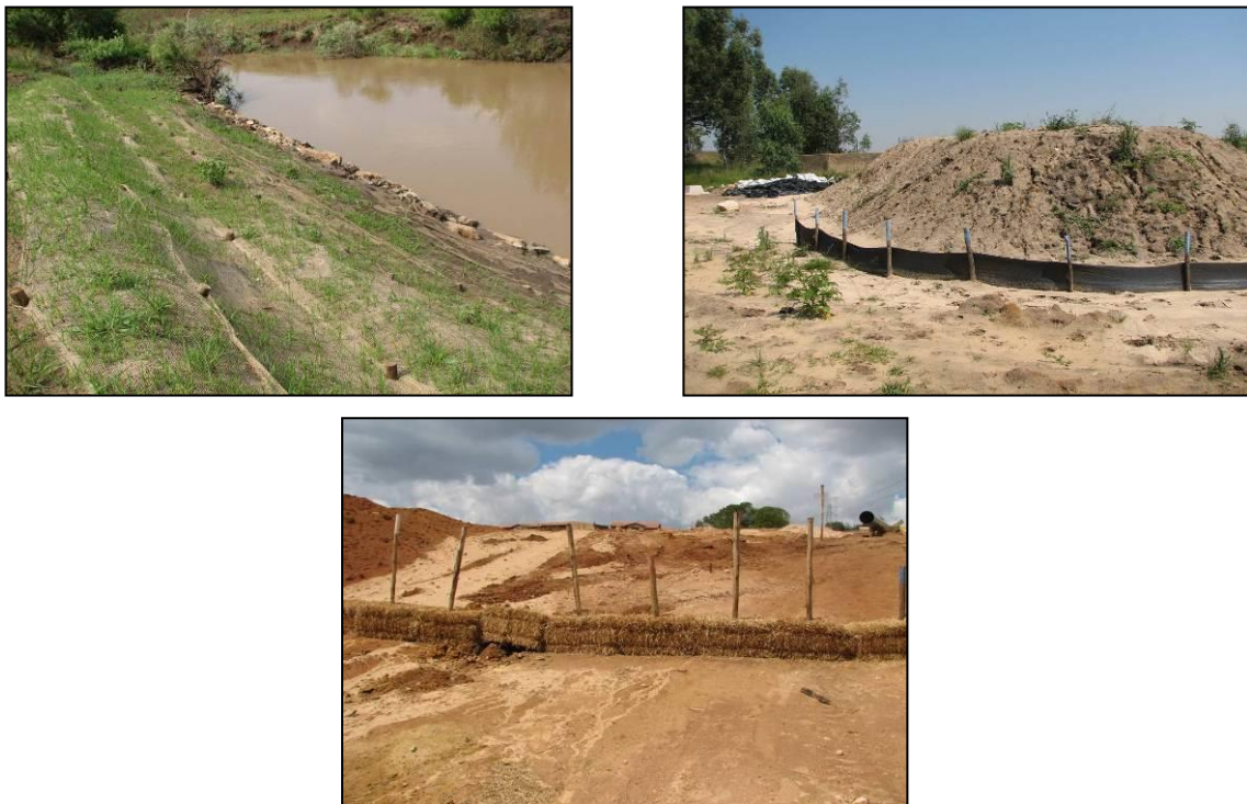
Figure 21: Typical soil erosion mitigatory measure: BioJute Installation ( top left ); a silt fence protecting a stockpile ( top right ) and pegged hay bale wall used to reduce runoff velocities ( bottom )
