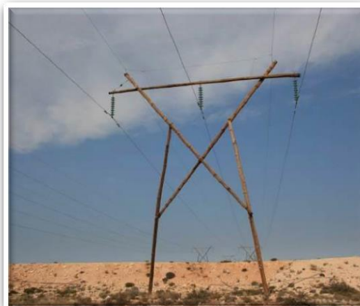
Example of an existing 132 kV transmission line (Source: Aurecon. 2013)
