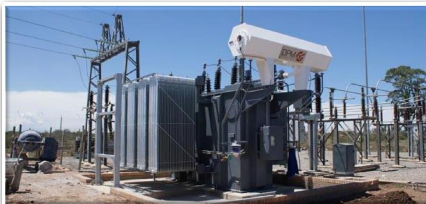
Substation with transformers at Sugarloaf Hill (Source: www.grocotts.co.za)
