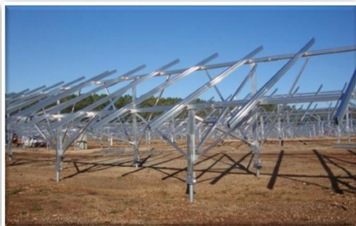
Photograph of example of mounting (Source: Provided by Aurecon)
