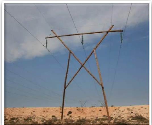
Example of an existing 132 kV transmission line (Source: Aurecon. 2013)
