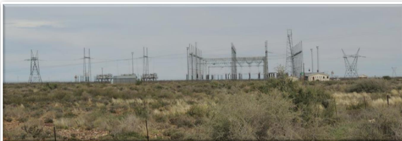
Figure 12: View of existing Cuprum substation
