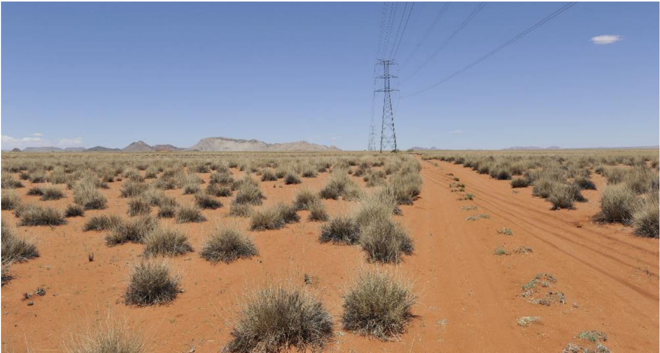
Figure 9: The Aggeneys - Harib 220kV transmission line runs through the assessment area.
