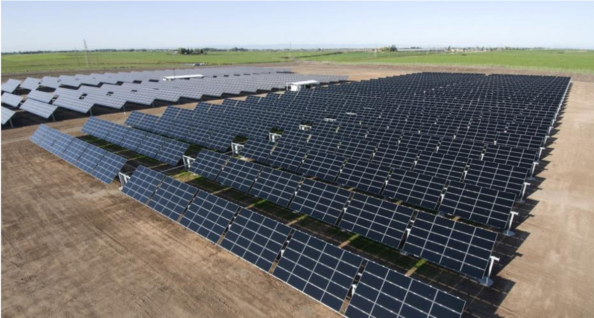
Figure 4: Photographic example of a Single Access Tracking PV technology (Solar Professional)
