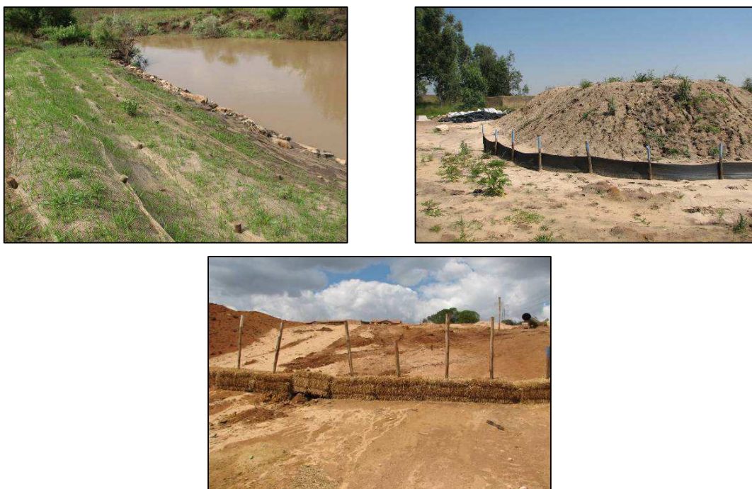
Figure 25: Typical soil erosion mitigatory measure: BioJute Installation ( top left ); a silt fence protecting a stockpile ( top right ) and pegged hay bale wall used to reduce runoff velocities ( bottom )
