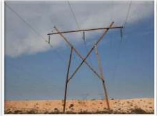
Example of an existing 132 kV transmission line (Source: Aurecon. 2013)
