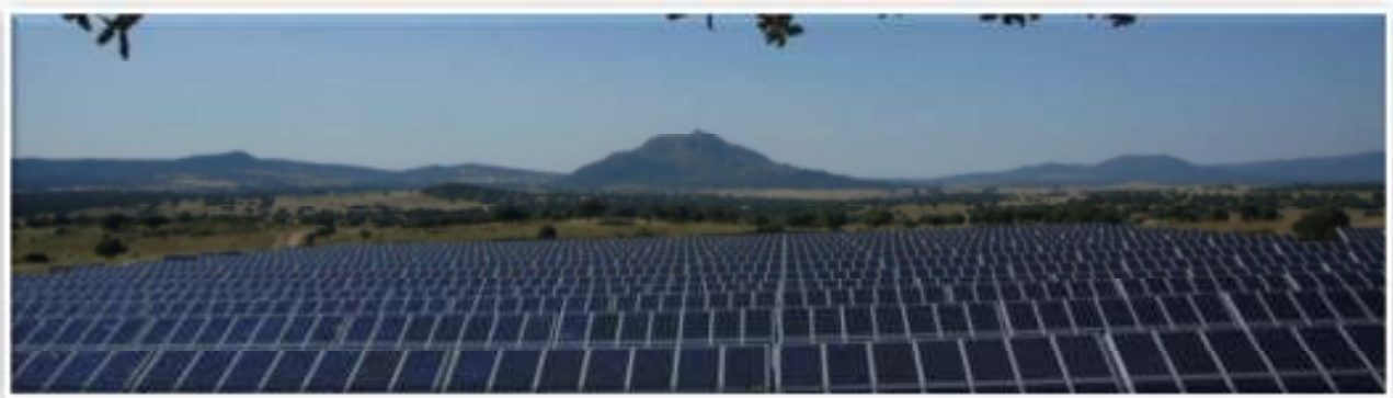
Example of solar plant (Source: www.hawaiiirenewableenergy.org/Villamesias2 )
