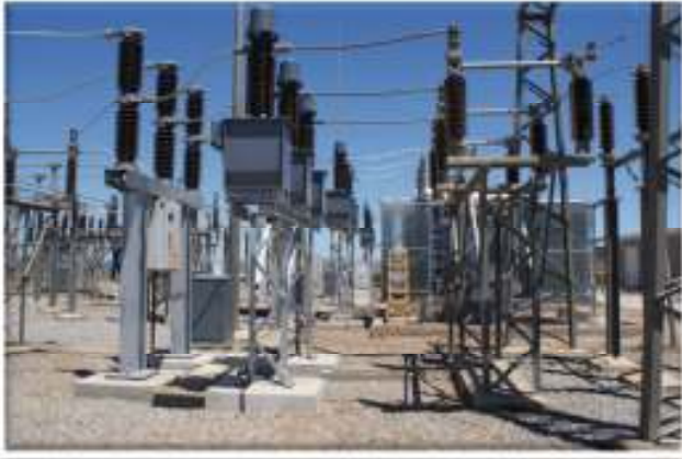
Substation with transformers at Sugarloaf Hill (Source: www.grocotts.co.za )
