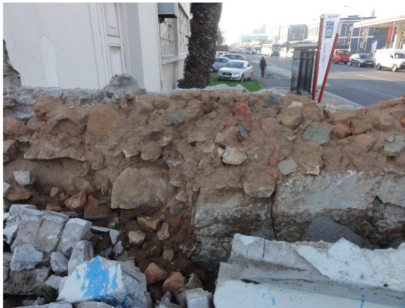
Fig 14 July 2018 wall collapse of eastern boundary wall.
