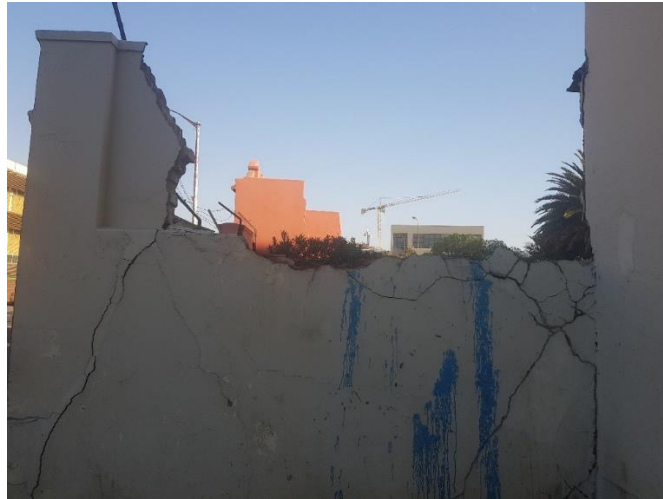
Fig 9. The collapsed lateral portion of the wall off Albert Road
