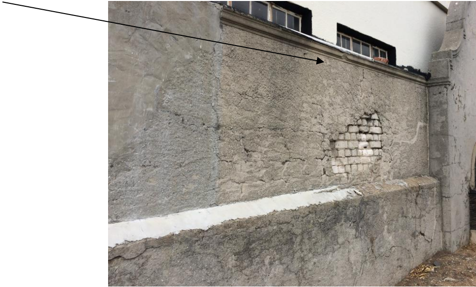
Fig 12 Wall along the eastern lateral boundary showing proximity to the adjacent building for the July 2018 collapse. June 2018
