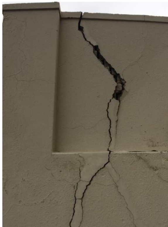
Fig 8. Cracks at the south eastern edge appearing before June 2018 Sections of this wall subsequently collapsed (see Fig 9)
