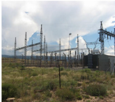
Figure 3: Drennan Traction Substation
