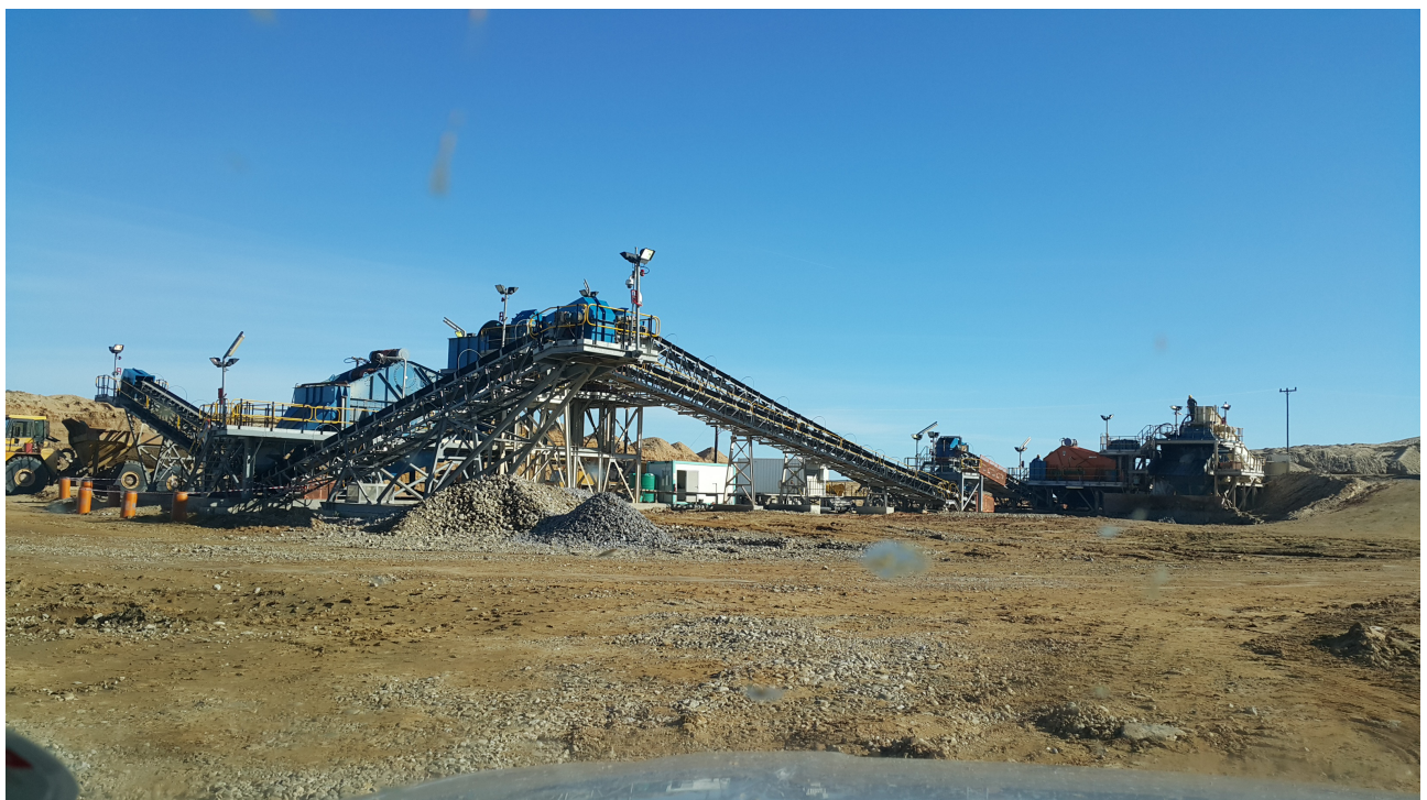
Figure 9.3 WCR screening and scrubbing plant near Koingnaas.
