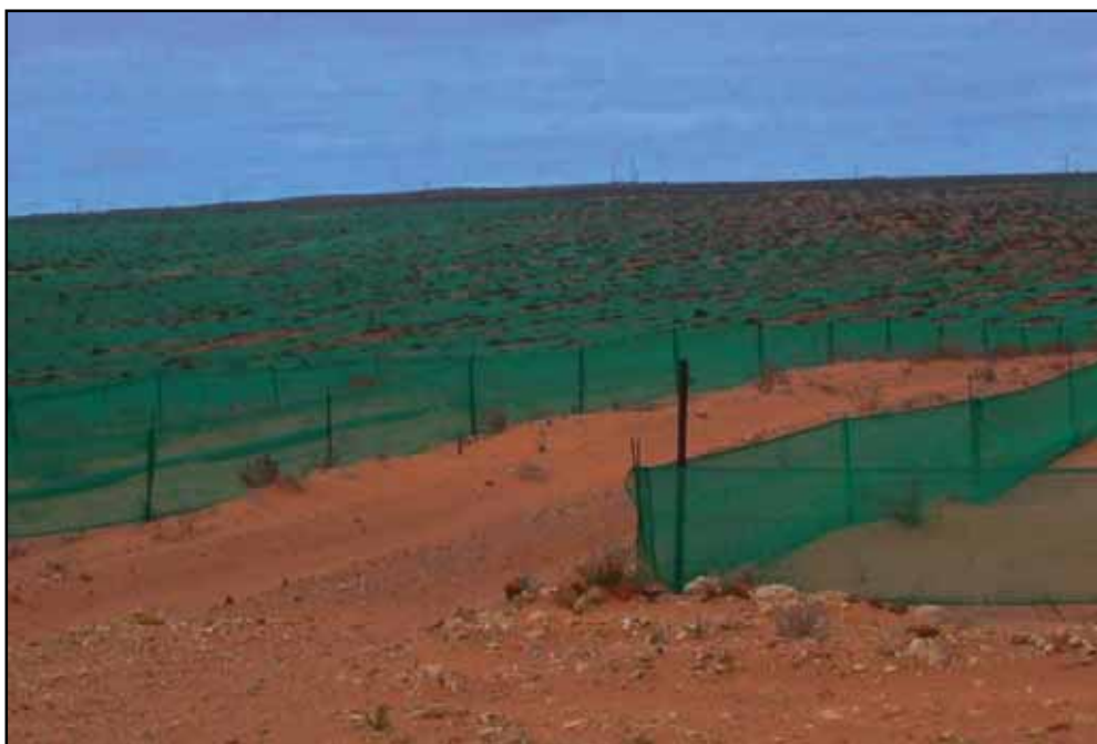
Plate 6. Rehabilitation underway at a mined area near to the site. The shade cloth barriers are to limit wind erosion and without them rehabilitation cannot take place due to sand movement which either smothers or erodes any seedlings being established. The image serves to illustrate the severity of wind erosion in the area and the extreme lengths that may be required to combat its' effects.
