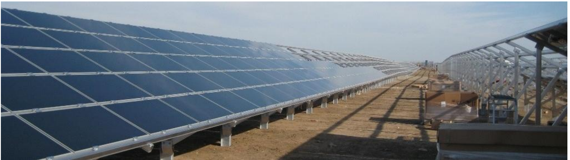
Figure 2: Photograph example of solar power panels (Source: ERM)
