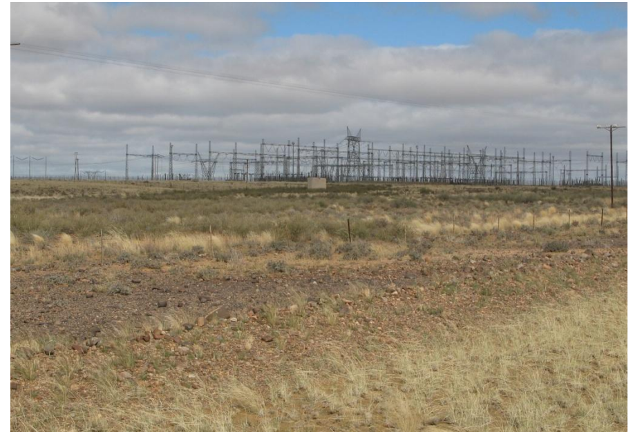
Figure 3: Aries sub-station (GPS 013)
