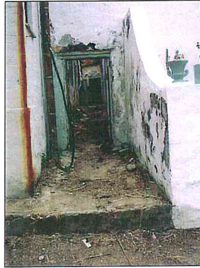
Fig. 20b. Passage to the back yard at the right hand side of 150 Buitengracht, 2007. At the back the toilets. The right hand passage wall dates from about 1770.
