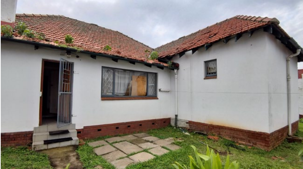
Figure 11. South West Elevation of the main dwelling. The extension to the main house in 1981 resulted in the roof structure having a pitch which is less than 17 degree. This has resulted in leaks through roof tiles. The ad hoc nature of the extension has also resulted in some awkward roof junctions.
