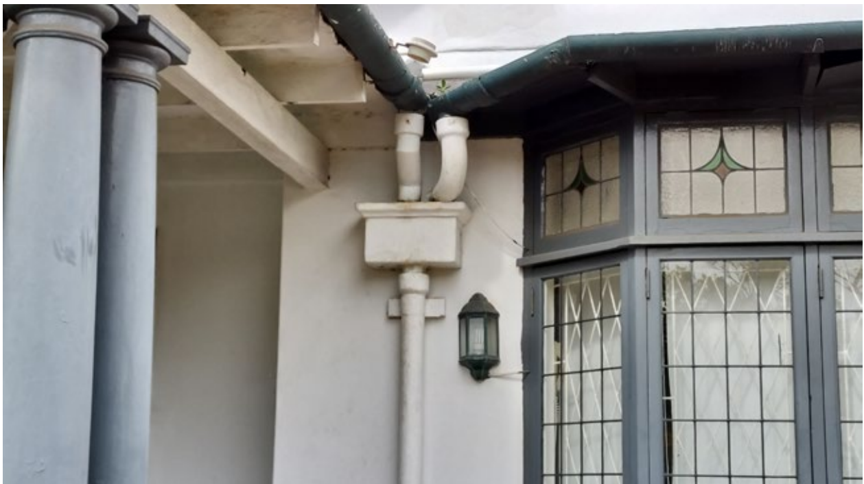
Figure 9. View of the verandah and bay window along the North East Facade. The bay window consists of lead light windows of which portions of the fanlight are stained glass.
