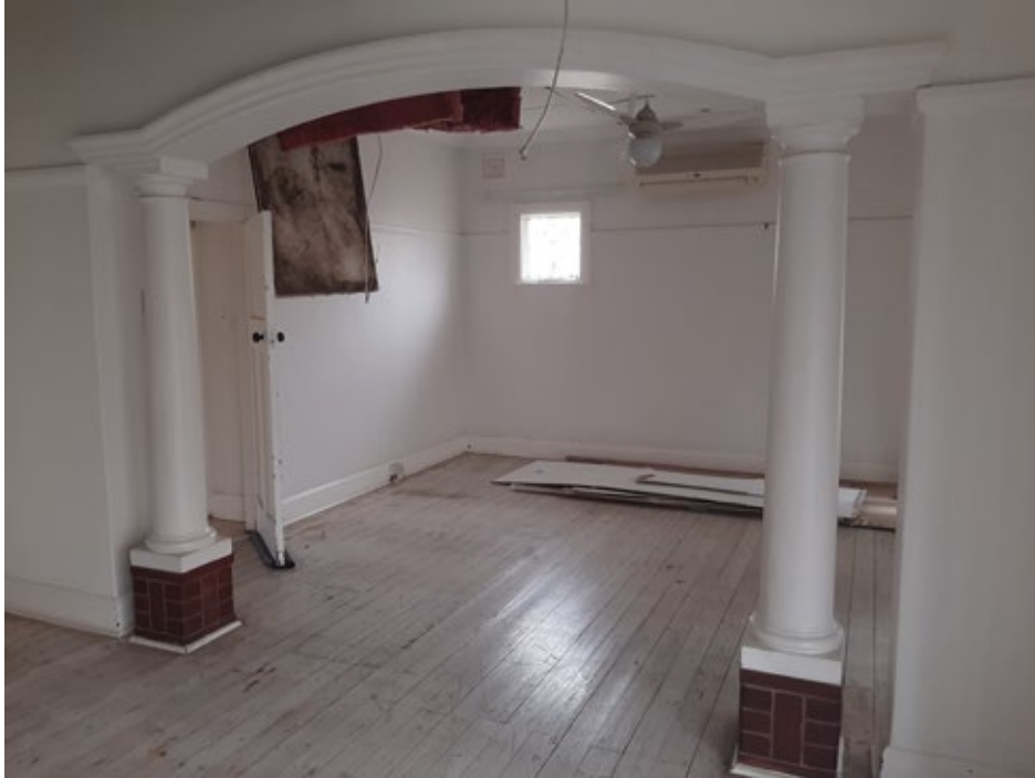
Figure 23. Internal view of lounge area. Painted timber suspended floors. Picture rails. Arched entrance to dining are framed by circular columns on red brick plinths.
