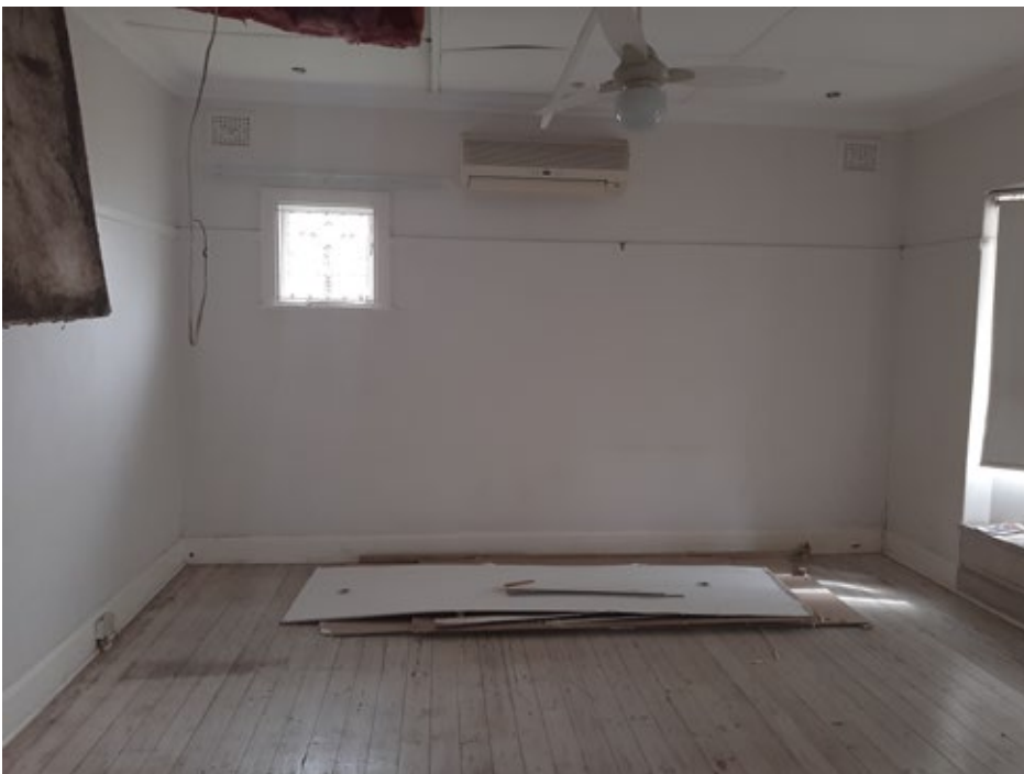
Figure 15. Internal view of the dining area. Painted timber suspended floors. Picture rails and a bay window.
