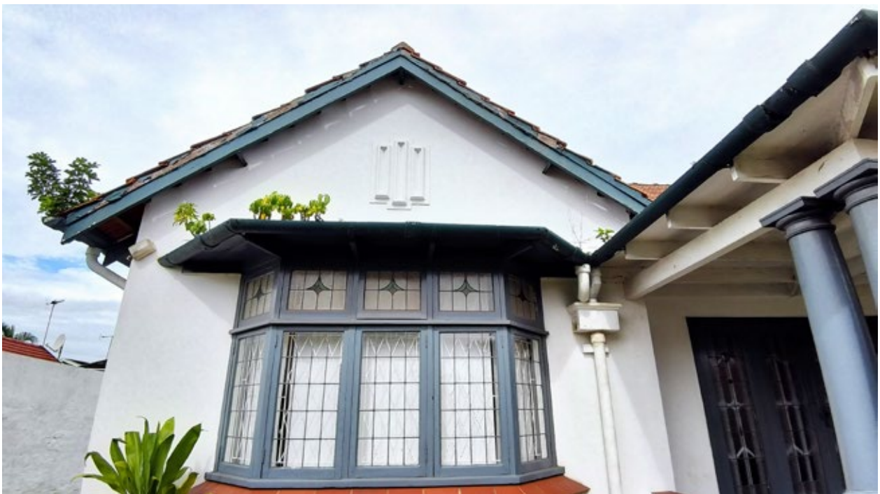
Figure 5. View of the a bay window on the North East Facade. Gable End roof above bay window.
