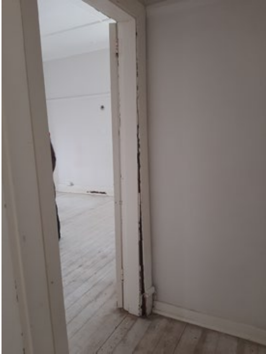
Figure 25. Internal view of passage showing borer infested door frame
