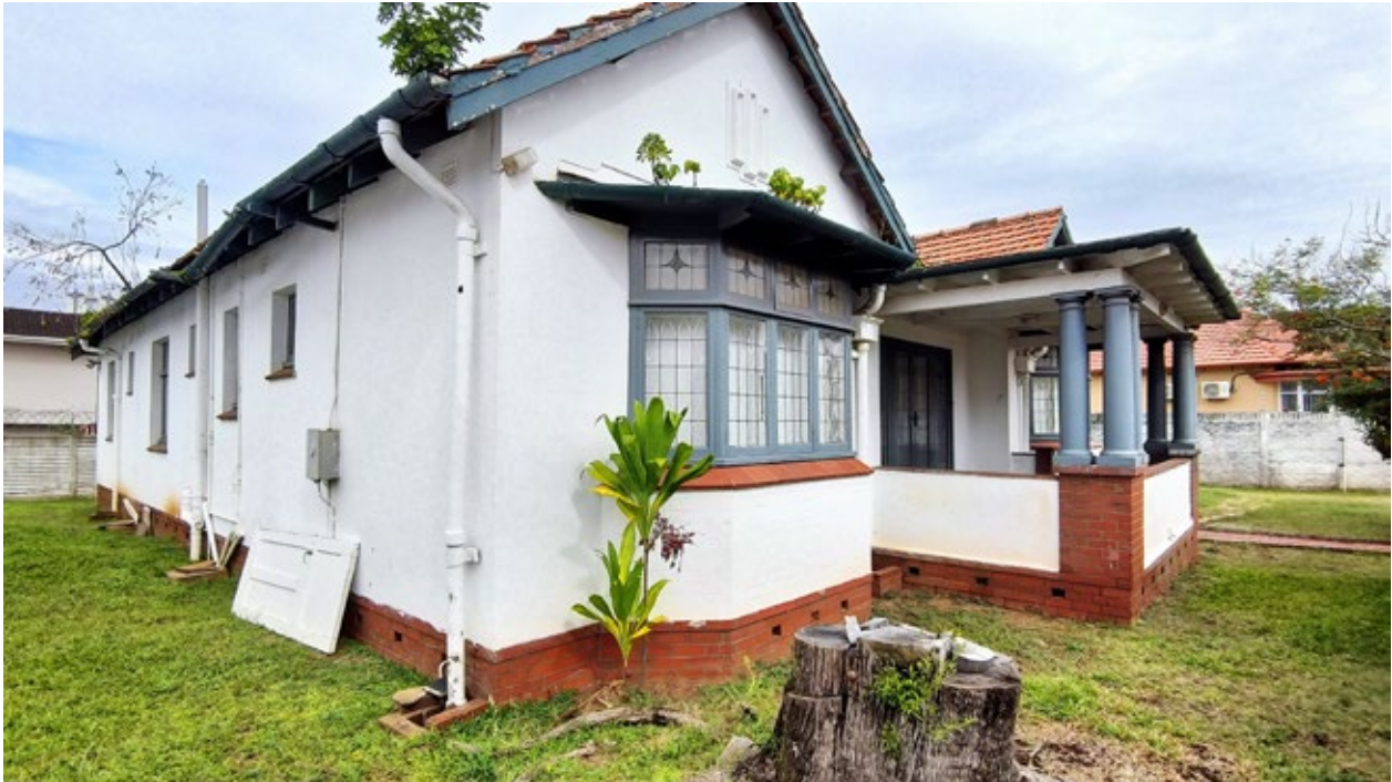
Figure 6. View of existing house from front garden showing the North East and South East facades. Red brick plinths. Smooth plastered walls. Gutters are damaged.
