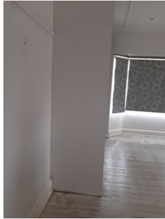
Figure 26. Internal view of main bedroom. Picture rails were not matched in areas where extensions were undertaken
