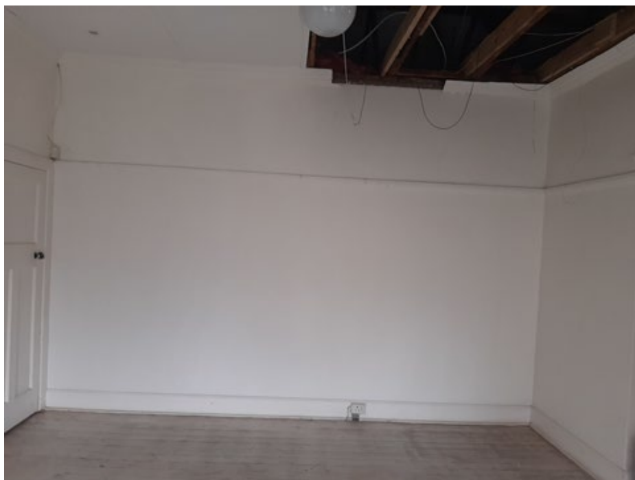
Figure 22. Internal view of bedroom. Contains picture rails. Ceiling has been removed to inspect roof trusses. Borer infestation confirmed and trusses in bad condition.
