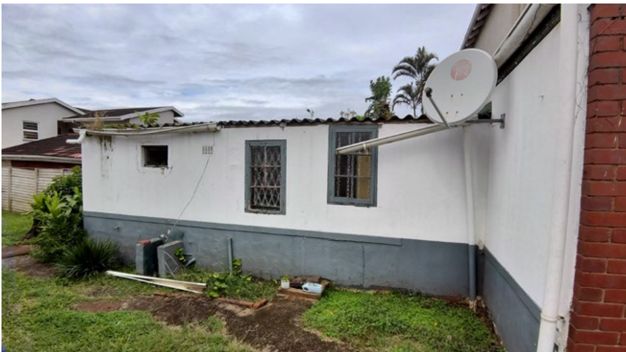
Figure 13. View of the outbuilding. Additions and Alterations were undertaken in 1981. Gutters have been badly damaged. Major cracking around small window. Plastered plinth is very reflects poor workmanship.
