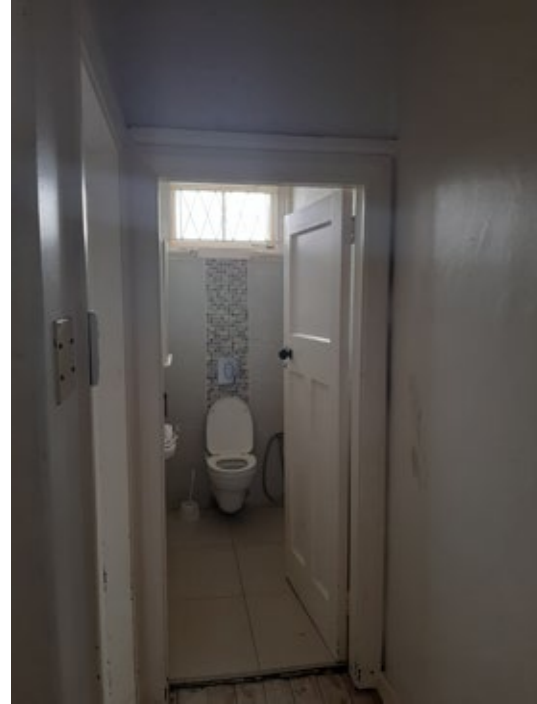
Figure 31. Internal view of wc. Has been recently revamped to a modern finish
