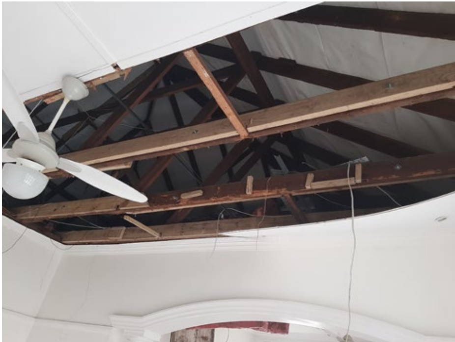
Figure 24. Internal view of lounge. Ceiling has been removed to inspect roof trusses. Borer infestation confirmed and trusses in bad condition. Repairs have previously undertaken
