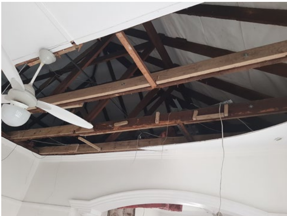
Figure 24. Internal view of lounge. Ceiling has been removed to inspect roof trusses. Borer infestation confirmed and trusses in bad condition. Repairs have previously undertaken
