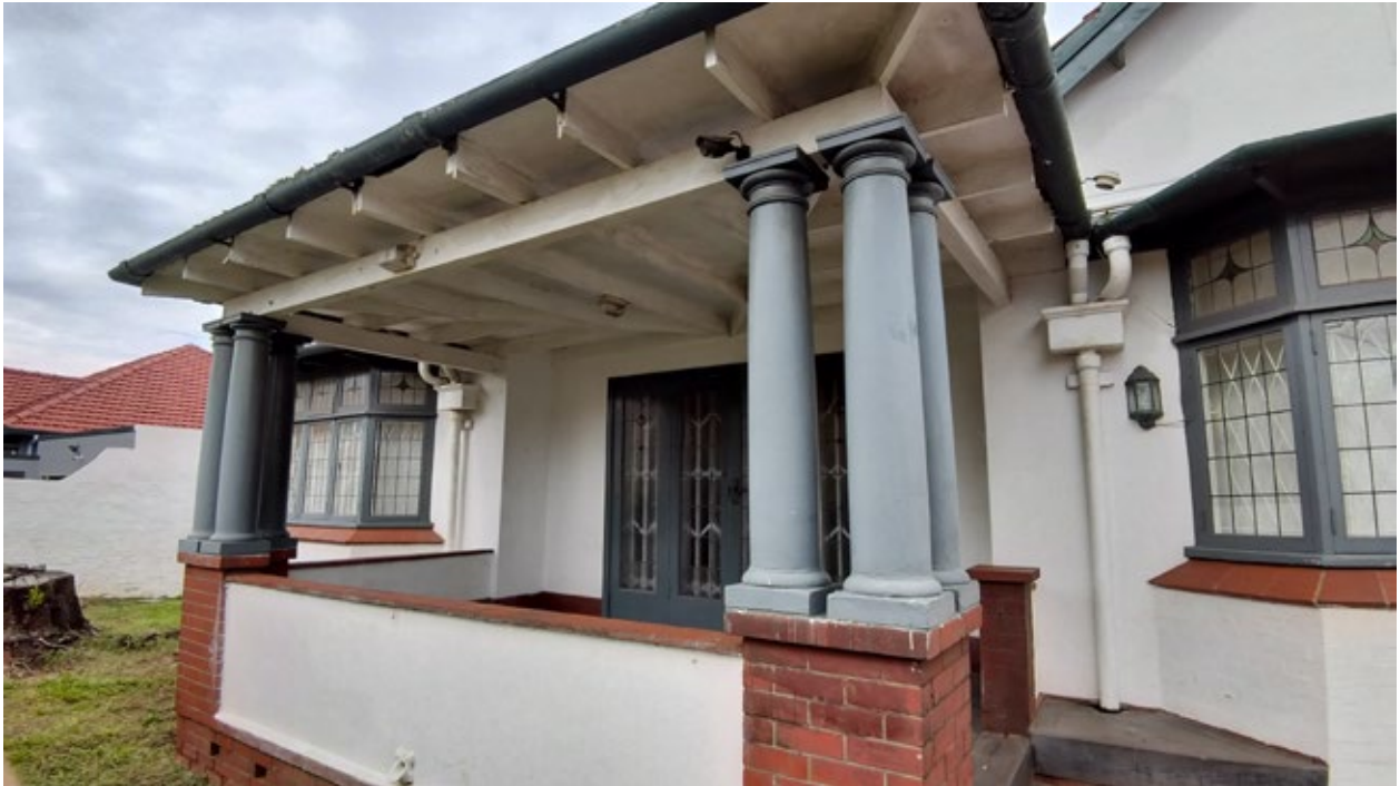
Figure 4. View of Verandah from front garden. Red brick Columns Plinths. Circular columns supporting Verandah roof structure.
