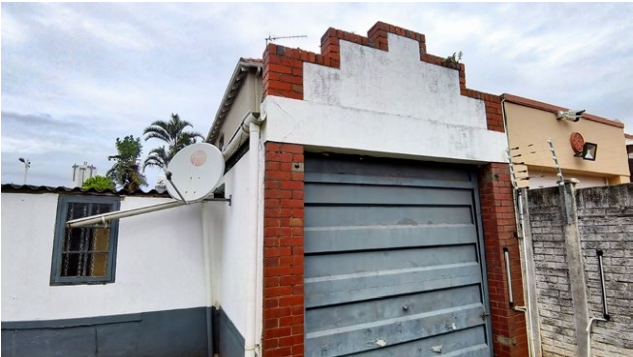
Figure 14. View of single garage from driveway. Consists of the red brick and plasters walls
