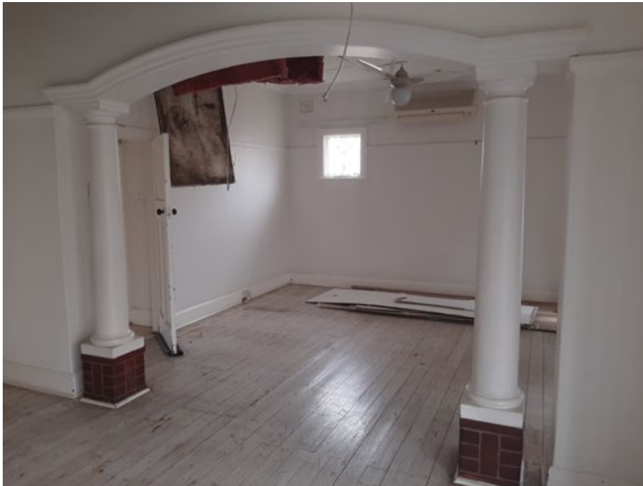
Figure 23. Internal view of lounge area. Painted timber suspended floors. Picture rails. Arched entrance to dining area framed by circular columns on red brick plinths.
