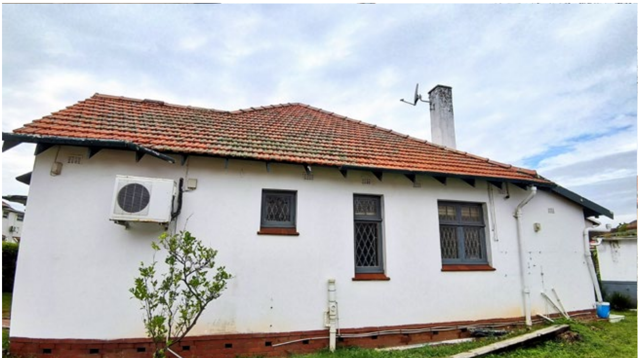
Figure 3. North West Elevation. Red Brick plinth. Smooth Plastered walls. Consists of timber windows. No significant architectural features or elements. Gutters have been damaged. Roof consists of marseille roof tiles
