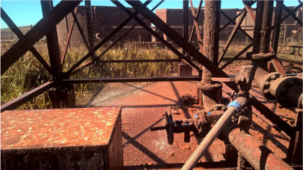
FIGURE 8: KING BRAITHWITE TANK LEAKING
