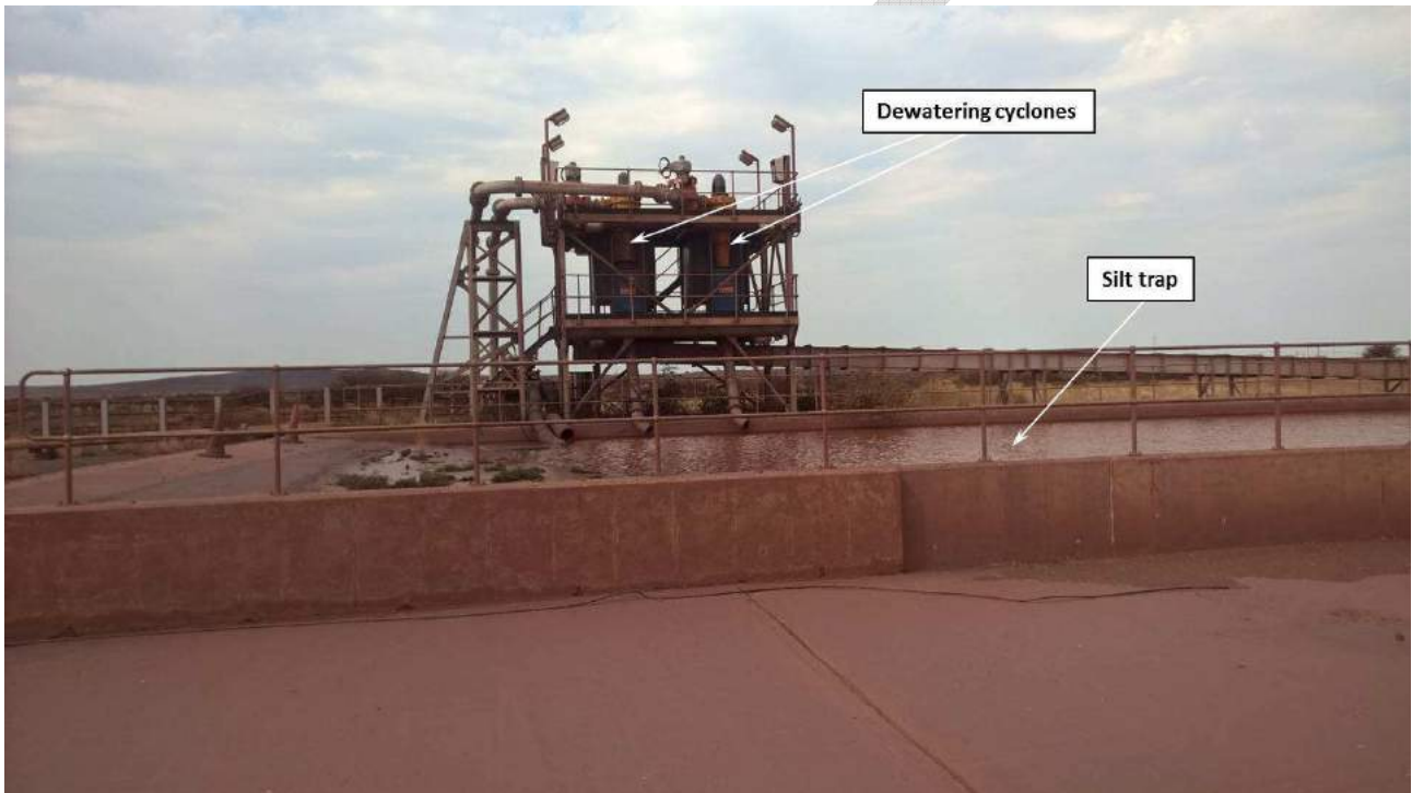
FIGURE 7: DEWATERING CYCLONES AND SILT TRAP AT THE PROCESS RECOVERY DAM
