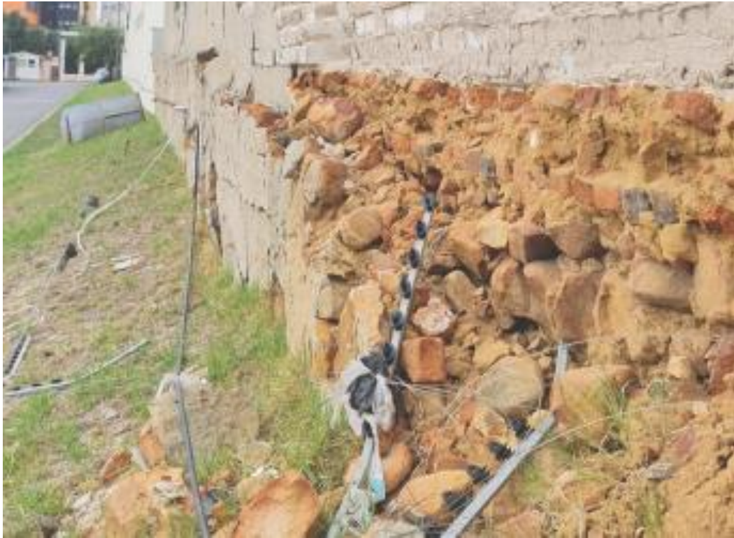
Fig 5. View of the northern wall collapse
