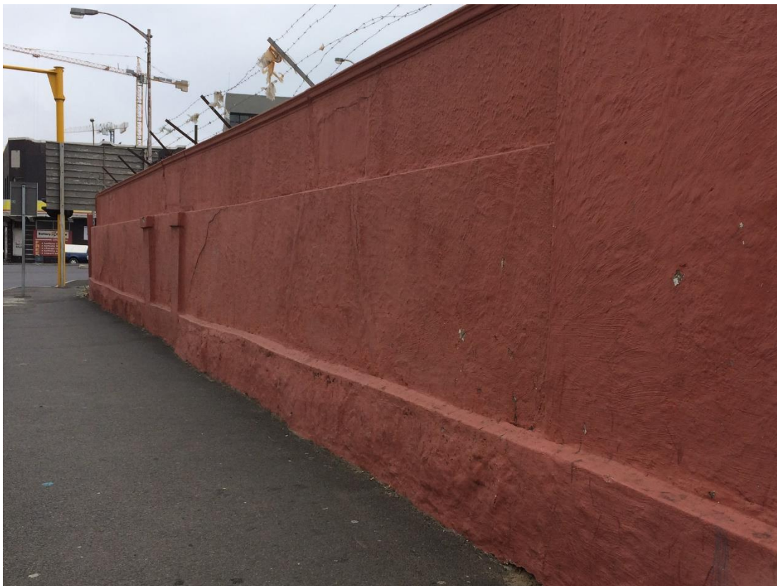
Fig 2. View along Albert Road towards the Lower Church Street Bridge and intersection
