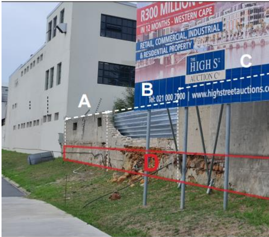
Fig 7. Wide view of the northern wall and building to the east of the cemetery showing mechanisms proposed to restore the wall.
