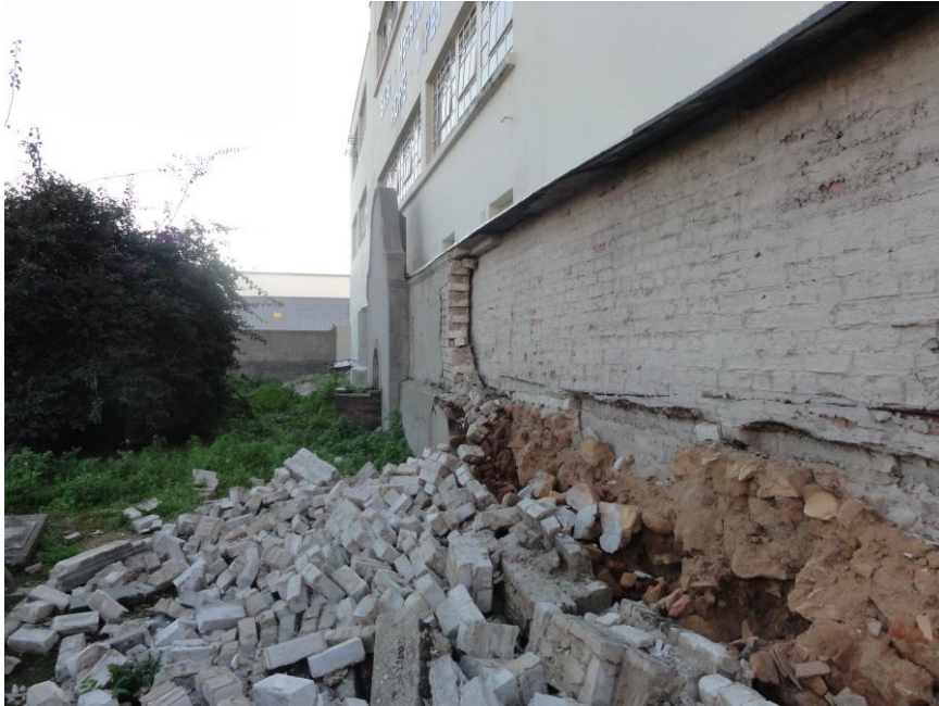
Fig 1. View of the eastern wall looking towards the northern wall. This show the collapse of the cement bricks built on top of the old stone wall. The cement bricks have been cleared.
