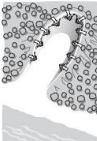
(a) Using earth moving equipment, push sand from blow-out lip into hollow.
