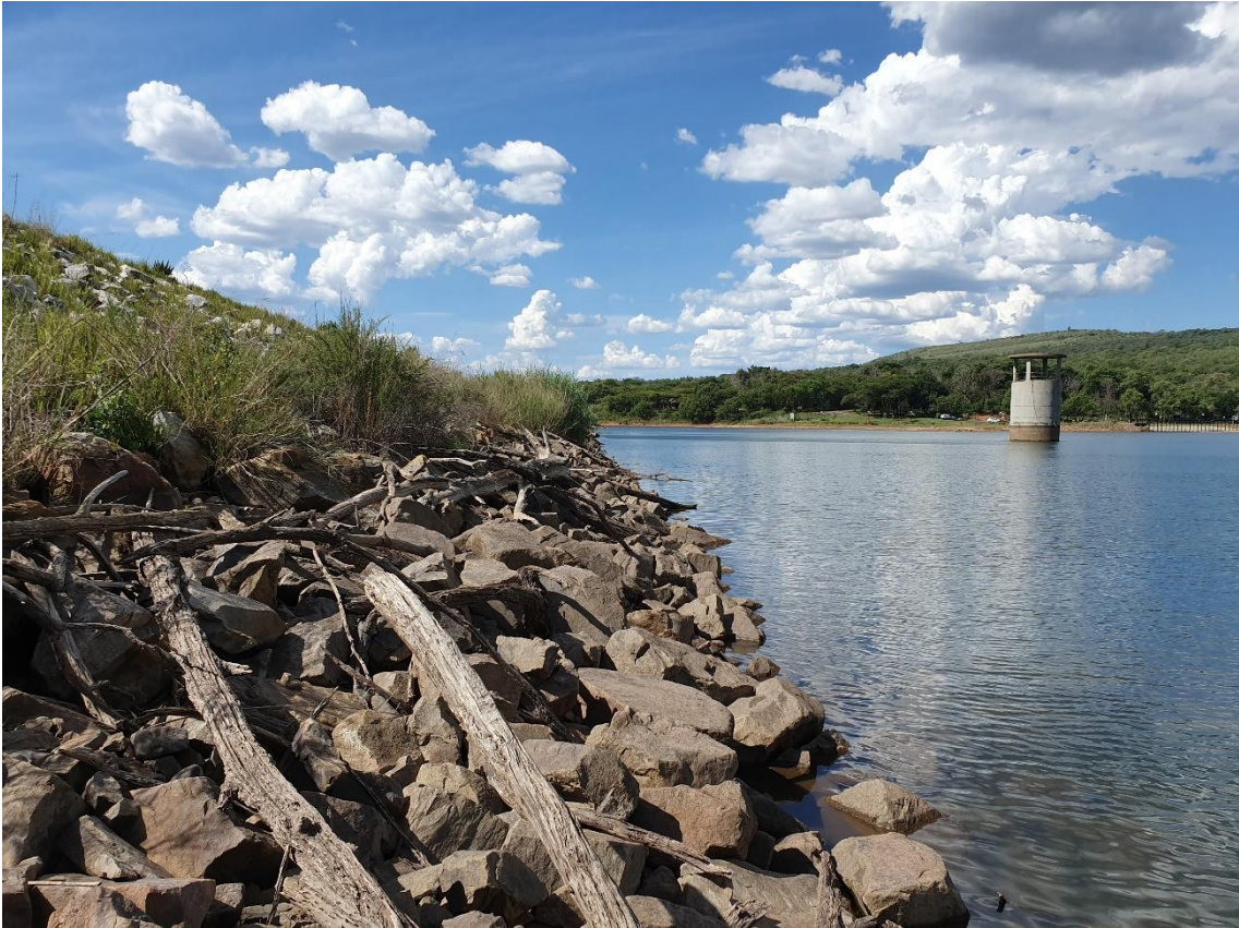
Photo 4: Lower upstream face of embankment showing good rip-rap upstream slope protection (19 November 2019).
