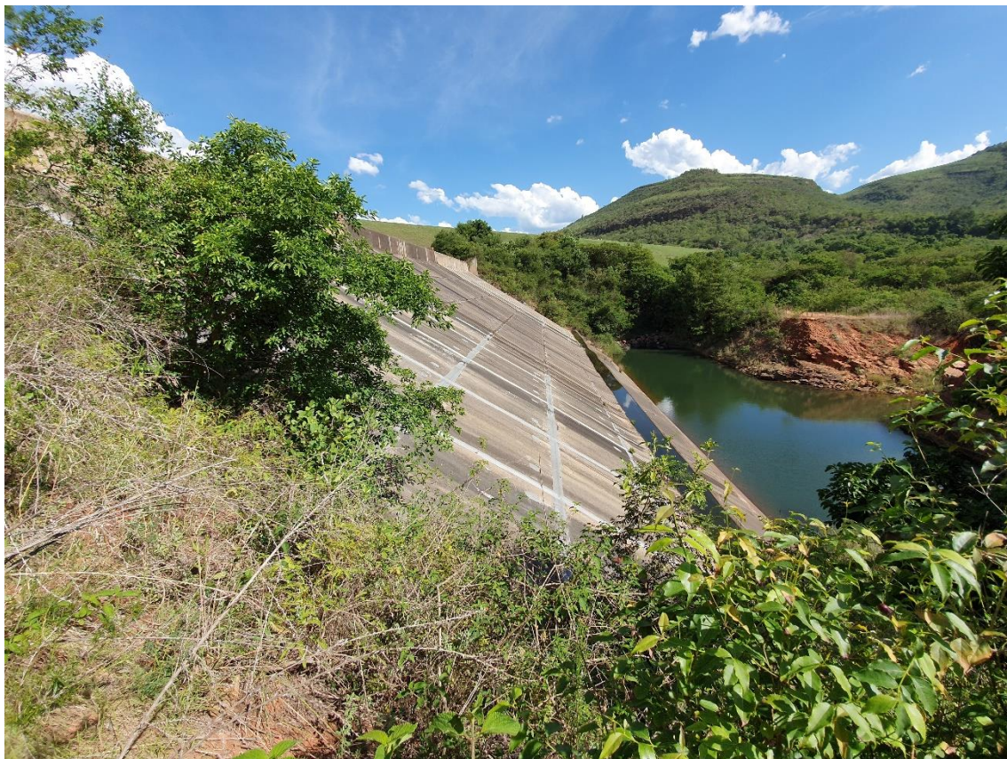
Photo 16: Spillway lower lining steep section (19 November 2019). Joint sealant also requiring repair.
