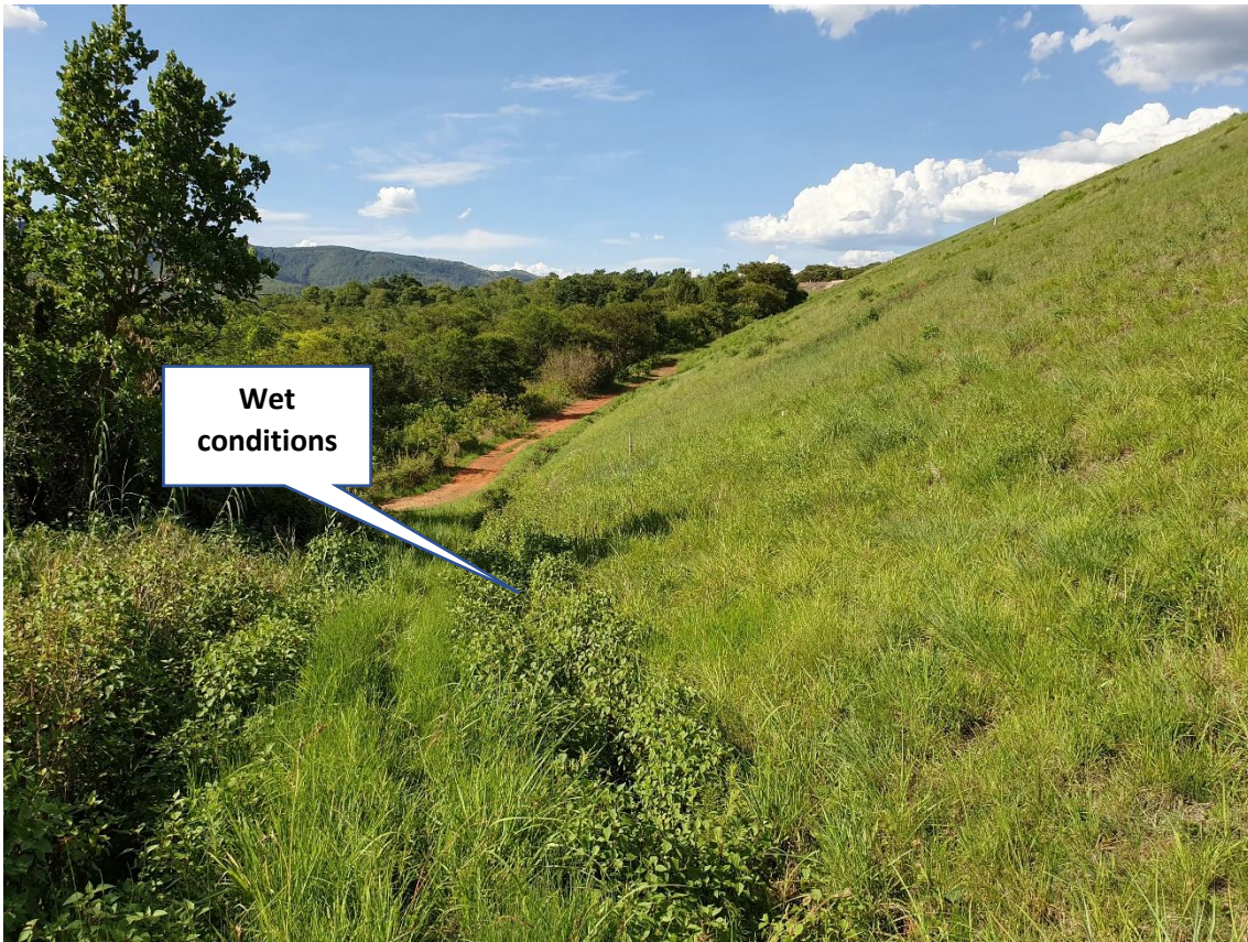
Photo 7: Downstream toe on lower left flank (19 November 2019). Note wet conditions which could be attributed to high phreatic surface within embankment.
