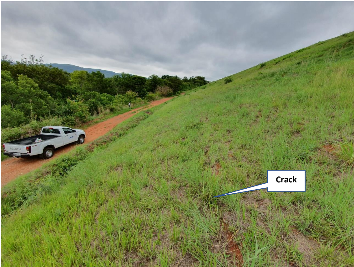
Photo 9: Downstream face from left flank (20 November 2019). Note longitudinal crack likely caused by surface slip movement.
