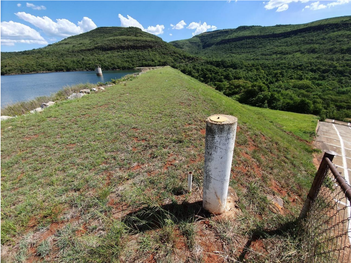
Photo 3: Embankment crest from end of right flank (19 November 2019). Note survey fixed station for movement monitoring.
