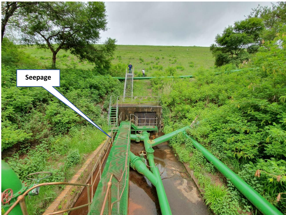
Photo 13: Outlet conduit exit at embankment toe (20 November 2019). Seepage was noted emanating from sides of conduit monitored at v-notch weirs.
