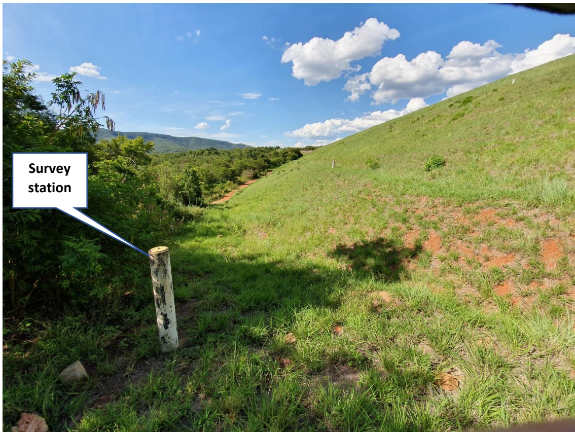
Photo 5: Lower downstream face from end of left flank (19 November 2019). Note survey fixed station for movement monitoring.
