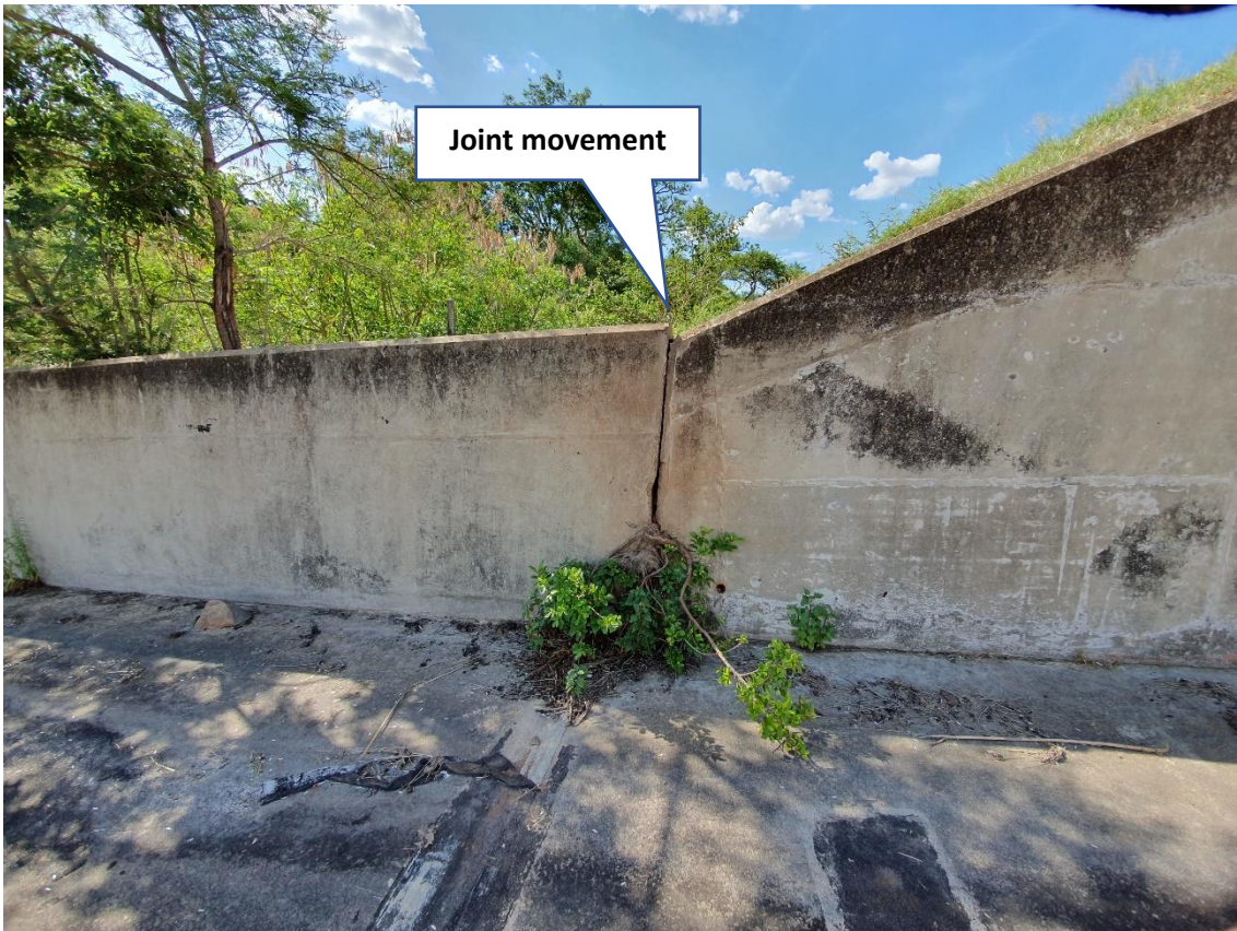
Photo 17: Spillway right training wall joint movement likely caused by tree roots (19 November 2019).
