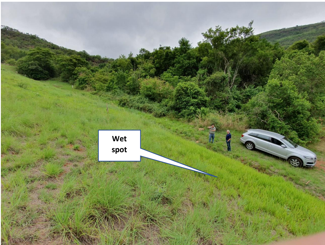
Photo 8: Downstream toe on lower left flank (20 November 2019). Note wet spot referred to in previous reports.
