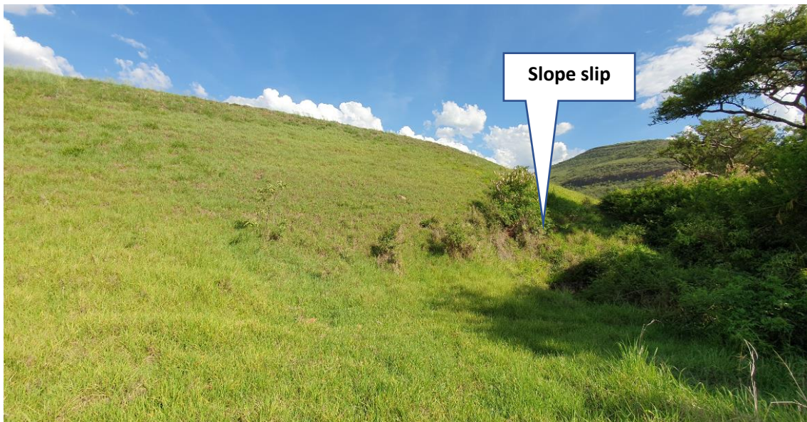
Photo 18: Downstream face of breaching section (fuseplug embankment) on right flank showing local slip (19 November 2019).
