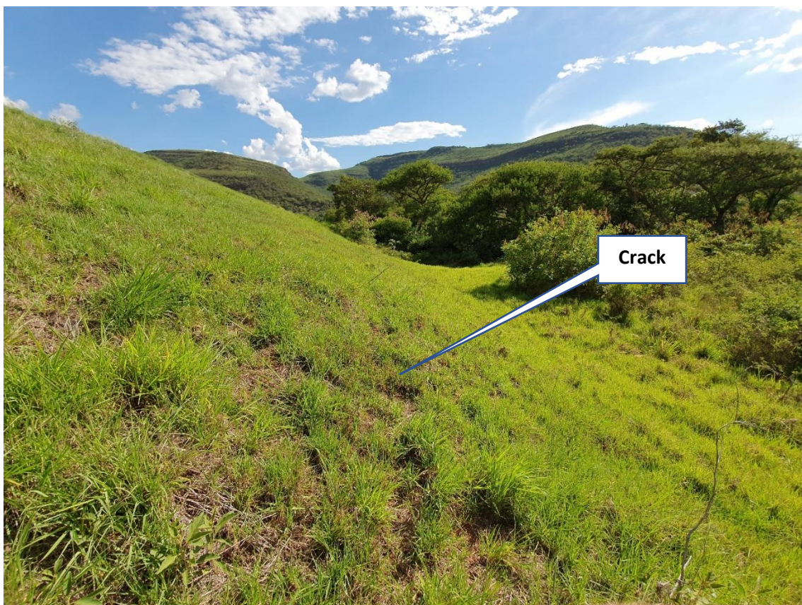
Photo 19: Breaching section downstream face towards left flank (19 November 2019). Note longitudinal crack likely caused by surface slip movement.
