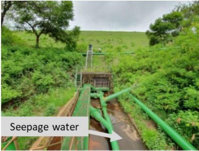
Figure 3: Outlet conduit exit at embankment toe (20 November 2019). Seepage was noted emanating from sides of conduit monitored at v-notch weirs.
