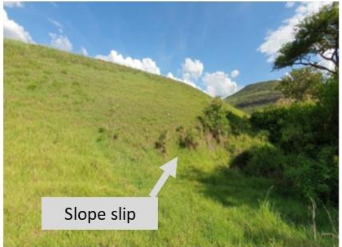
Figure 6: Downstream face of breaching section (fuseplug embankment) on right flank showing local slip (19 November 2019).
