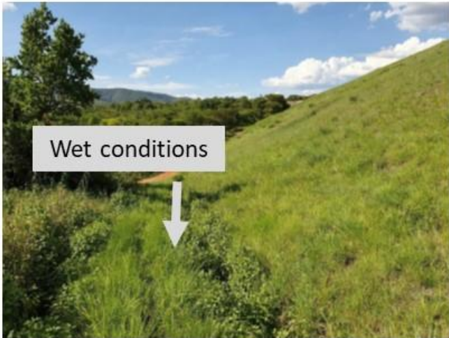
Figure 5: Downstream toe on lower left flank (19 November 2019). Note wet conditions which could be attributed to high phreatic surface within embankment.
