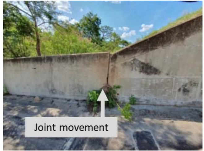
Figure 4: Spillway right training wall joint movement likely caused by tree roots (19 November 2019).
