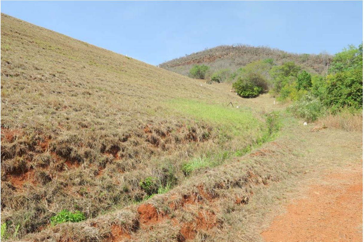
PLATE 11:- Wet spot (green grass) near bottom of embankment at left flank
