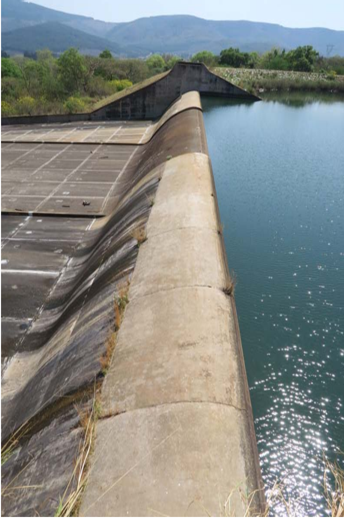
PLATE 9:- Spillway OGEE control structure - grass growing in construction joints
