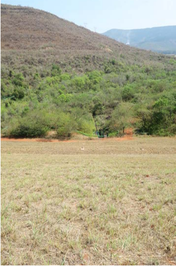
PLATE 5:- Standpipe piezometers SP1-3 along “culvert” section
