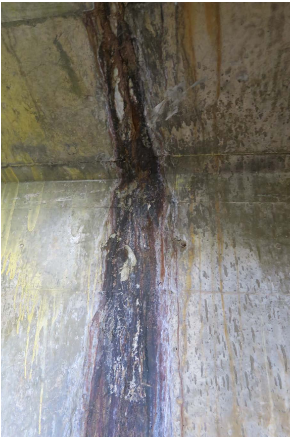
PLATE 14:- material seeping into outlet conduit at CH 106 (as measured from inside face of outlet tower in downstream direction).
