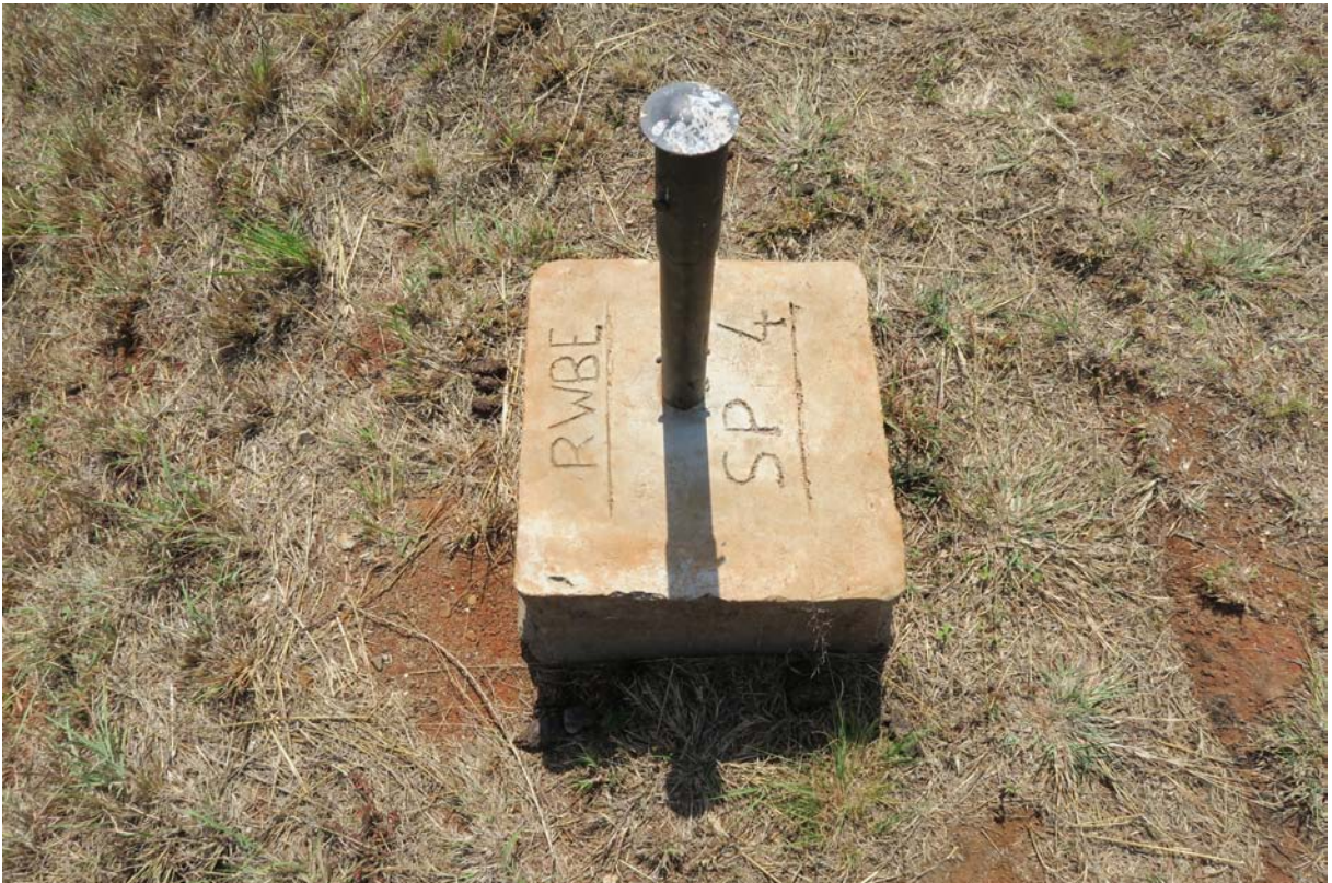
PLATE 2:- Standpipe piezometer SP4 on dam crest at “riverbed” section.
