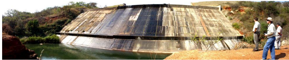
Plate G9. View of spillway. Note that curved appearance is due to "photo stitching".
