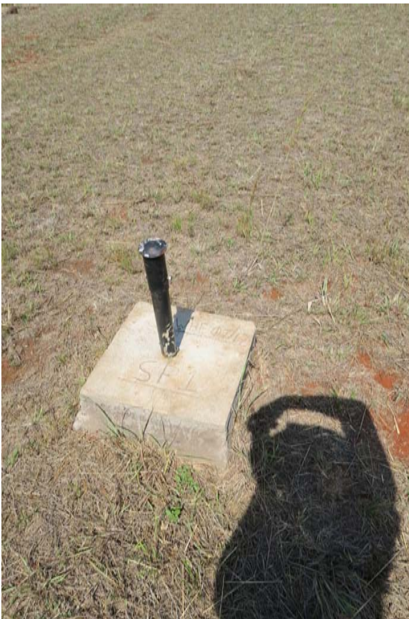
PLATE 4:- Standpipe piezometer SP1 on dam wall crest at “culvert” section
