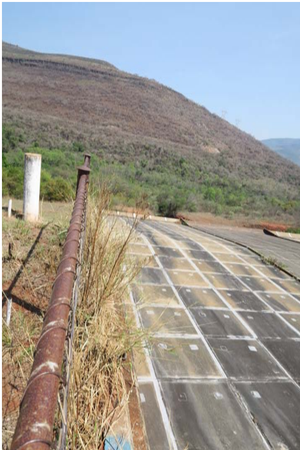
PLATE 6:- Spillway return channel and “bandaging” of joints
