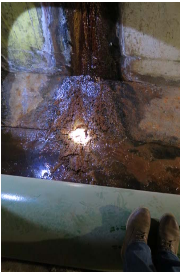
PLATE 16:- material seeping into outlet conduit at CH 63 (as measured from inside face of outlet tower in downstream direction).
