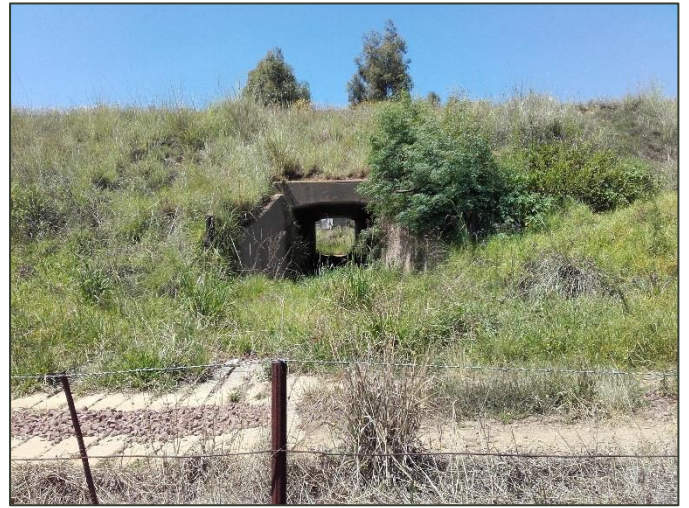
Figure 2: Underground train bridge south-west of the proposed development, proposed for pedestrian access
