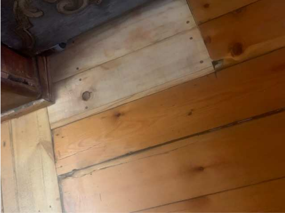
Floor boards have been patched up in places where it was untrafficable.
