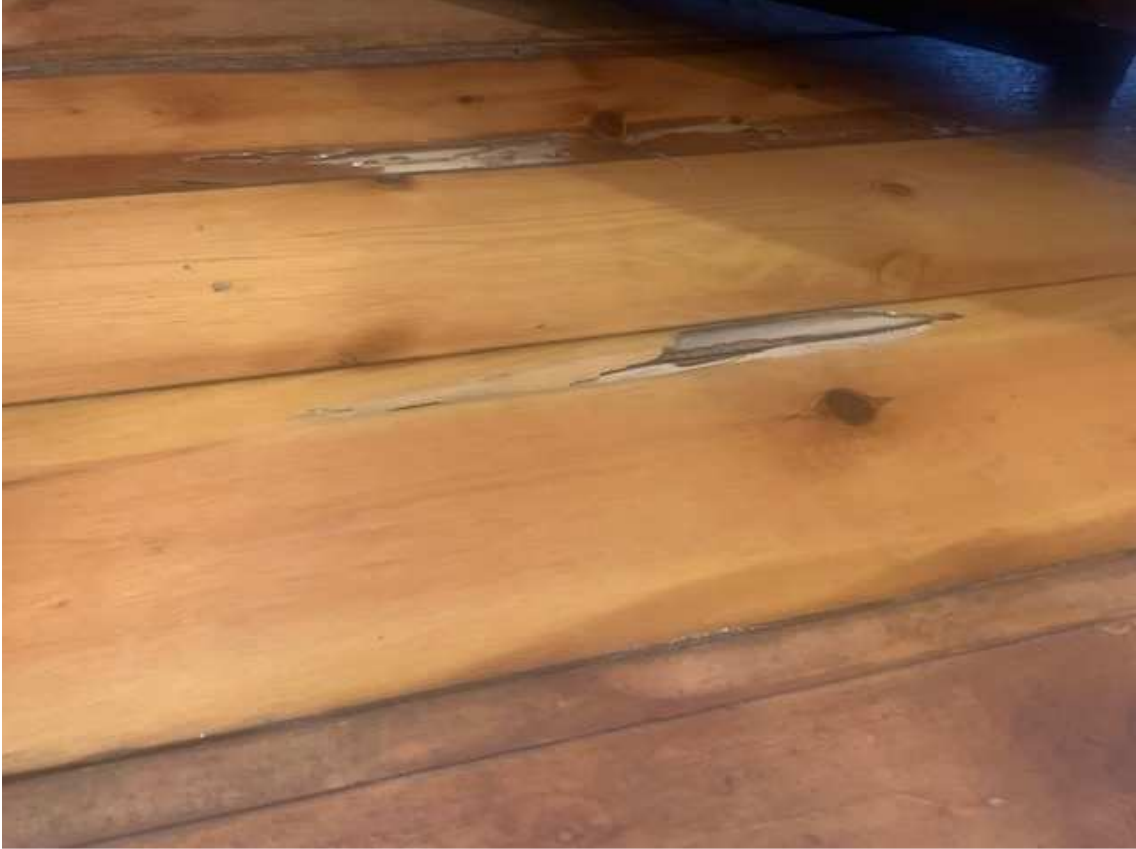
Wood borer have eaten through the existing floor boards in places, breaking as they are stood on.
