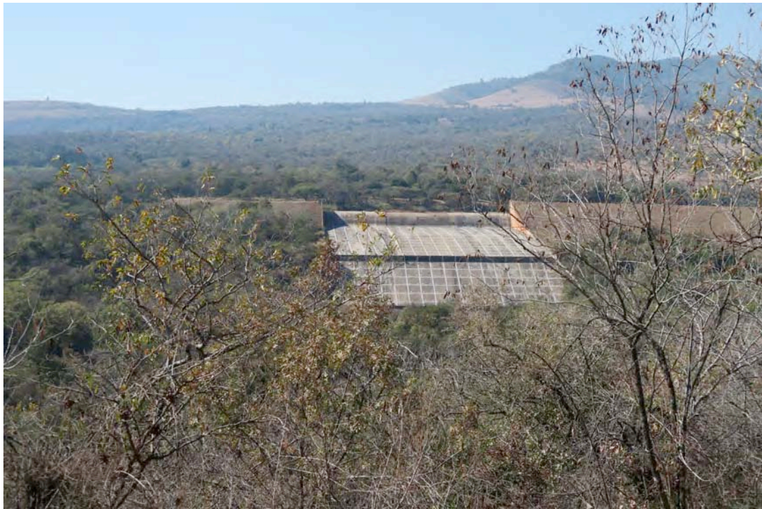
Plate 11:- View of spillway control structure and return channel – Note repair bandages over construction joints (2016-07-12)
