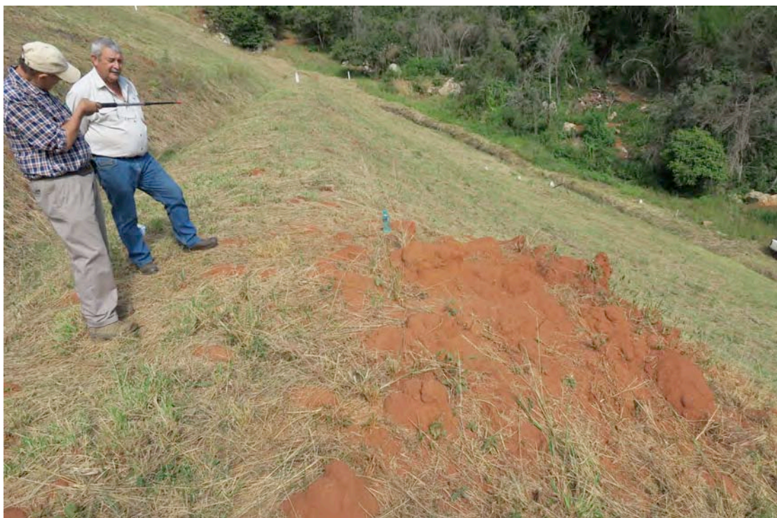
Plate 24:- Termite activity near left flank upper berm (2016-05-10)
