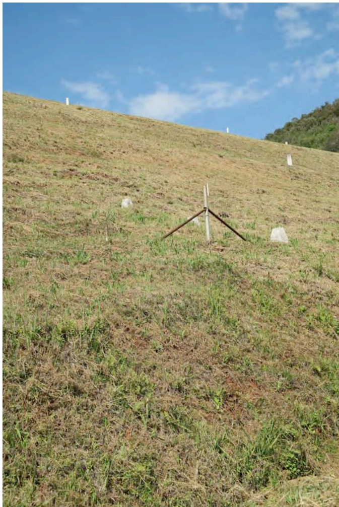
Plate 14:- Survey beacons at “wet spot” on embankment slope near left flank. The “wet spot” was dry at time of inspection. (2016-05-10)
