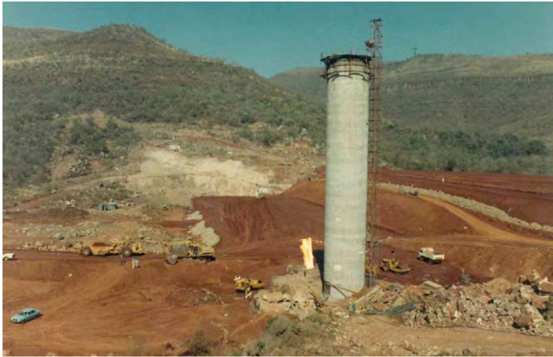
Plate 3:- View towards left flank, showing partly constructed embankment and exposed left bank foundations comprising a cover of partly recemented (calcified) talus blocks in a matrix of soil, resting upon a layer of completely weathered very weak tuff and agglomerate
