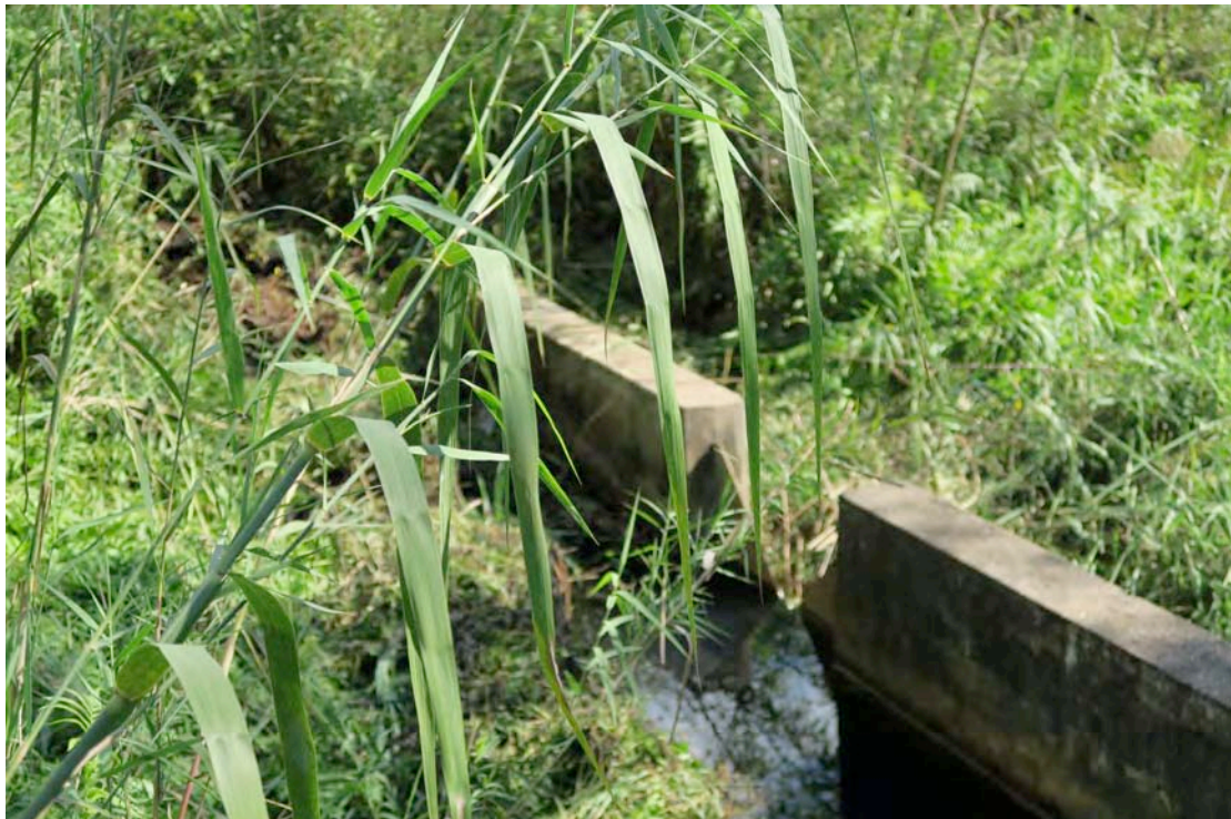
Plate 18:- “Seepage 1” v-notch gauge in old river bed – to be discontinued due to ingress of other seepage, i.e. not from “dam” seepage (2016-05-10)
