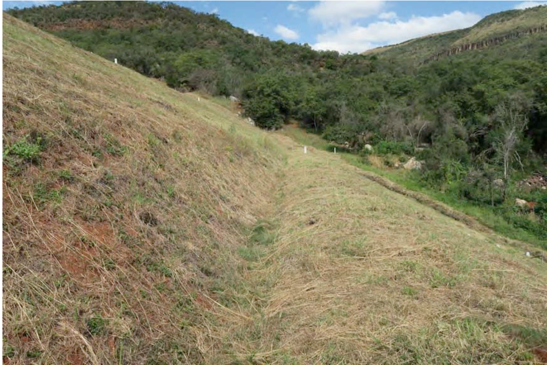
Plate 15:- Survey beacons (top left and bottom right). Faulty piezometers on berm (centre of picture). (2016-05-10)
