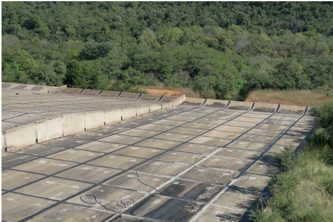
Plate 10:- Service spillway return channel with “kink” and “flip bucket”. Note new repair bandages over construction joints. (2016-05-10)
