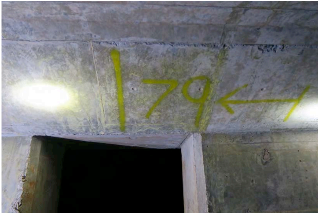
Plate 21:- Outlet conduit:- left-side compartment, right wall, 79 m from intake tower:- access opening into right-side compartment (2016-07-12)
