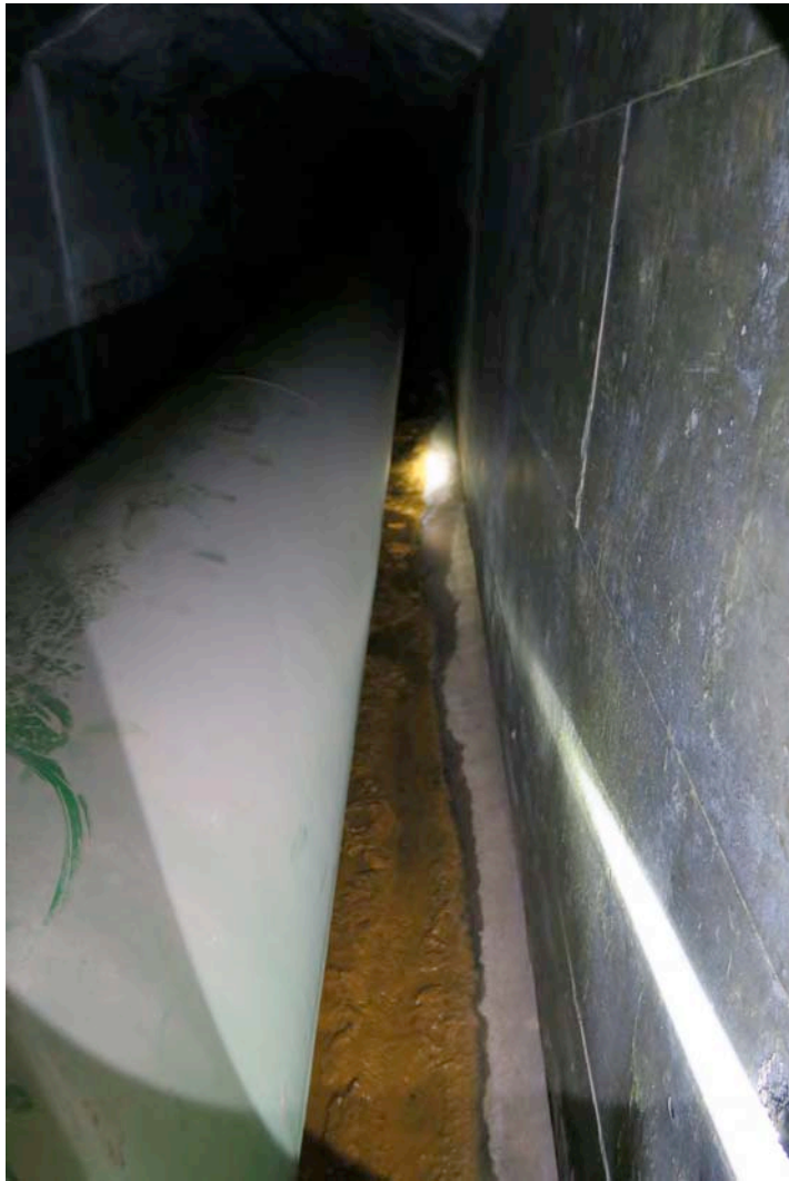
Plate 23:- Outlet conduit:- right-side compartment floor, 66 m from intake tower:- upstream view of seepage of embankment material down the conduit floor (outlet pipe on left and dividing wall on right) (2016-07-12)
