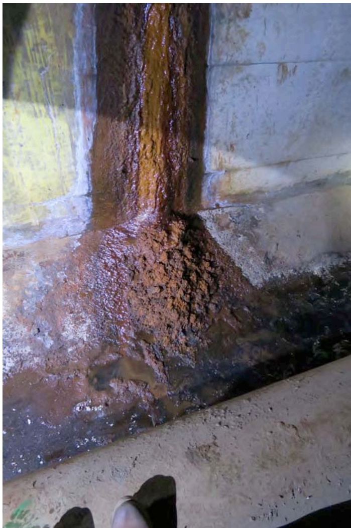
Plate 22:- Outlet conduit:- right-side compartment, right wall, 66 m from intake tower:- seepage of embankment material through construction joint (2016-07-12)
