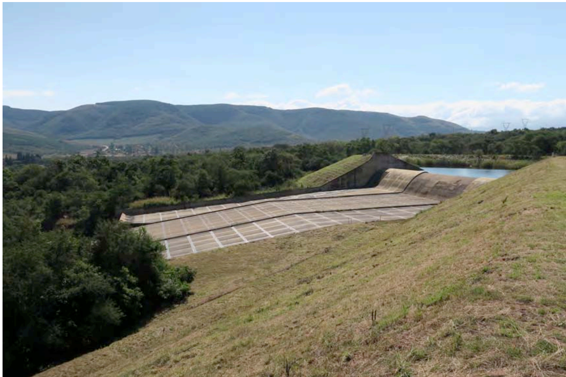
Plate 8:- View from left bank with emergency breaching section in far right background (2016-05-10)
