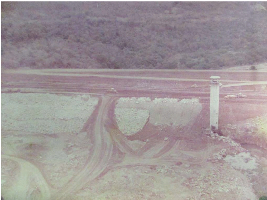
Plate 4:- Downstream view from inside dam basin. Note rock cuts adjacent to inlet tower indicating good founding conditions.
