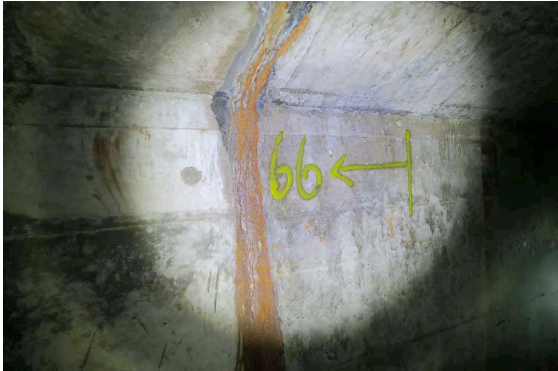
Plate 19:- Outlet conduit:- left-side compartment, right wall, 66 m from intake tower:- seepage of embankment material through construction joint (2016-05-10)
