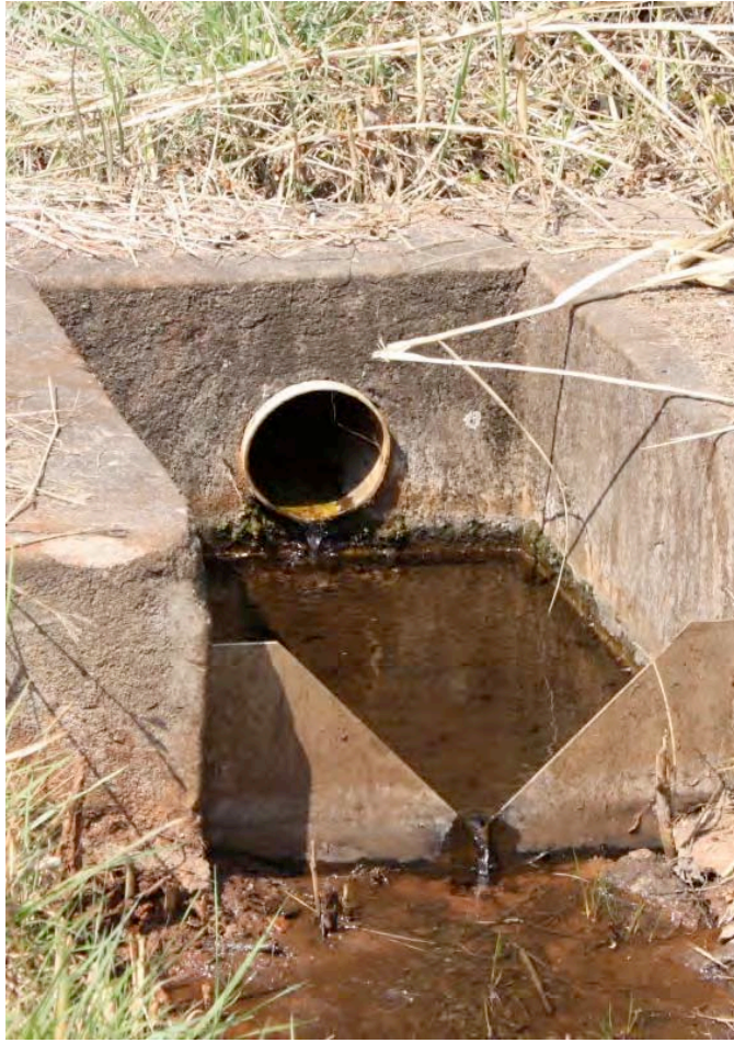
Plate 17:- V-notch gauge at outlet for combined “toe-drain East and toe-drain West” (2016-05-10)
