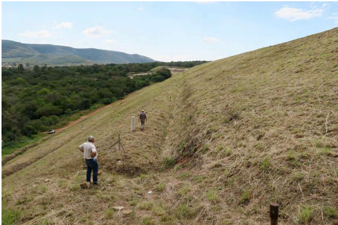
Plate 16:- Faulty piezometers on berm to be replaced with new standpipe piezometers (2016-05-10)
