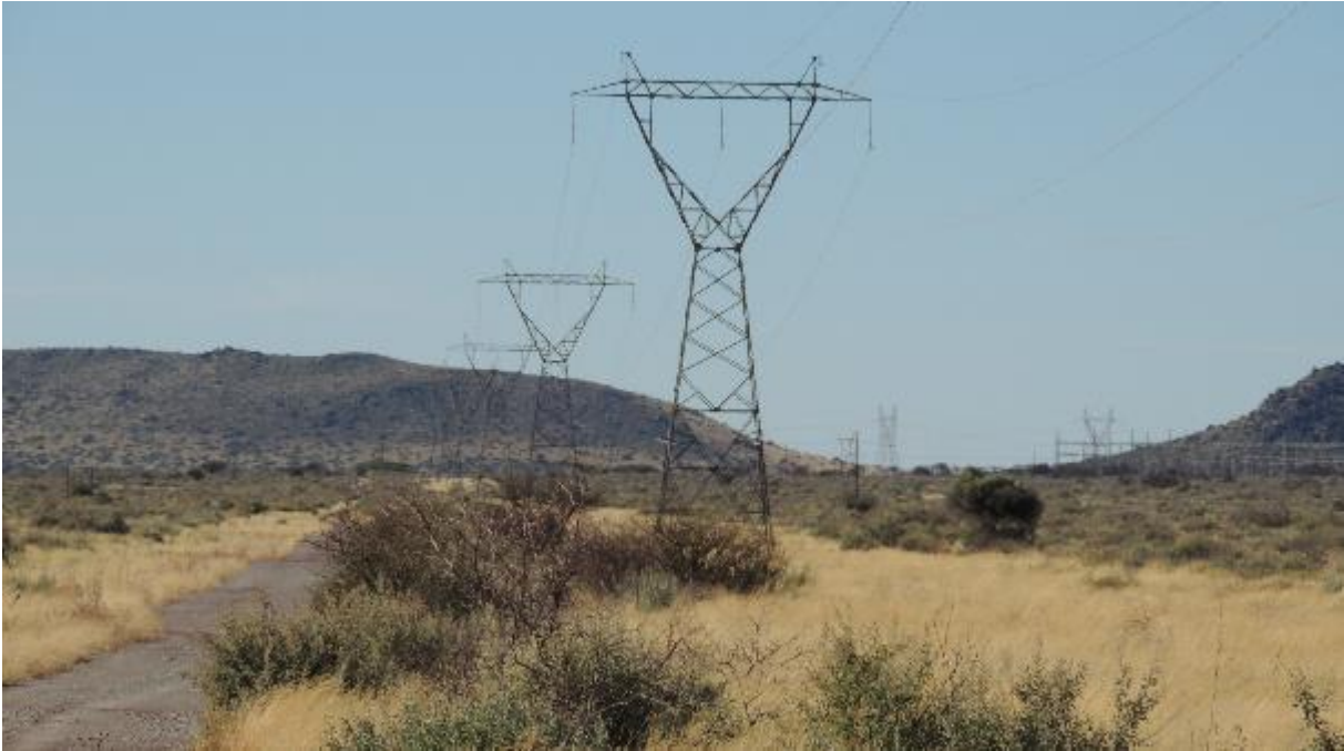
Figure 11: Photograph of the existing Eskom 132kv powerline and the small substation located to the east of the project site
