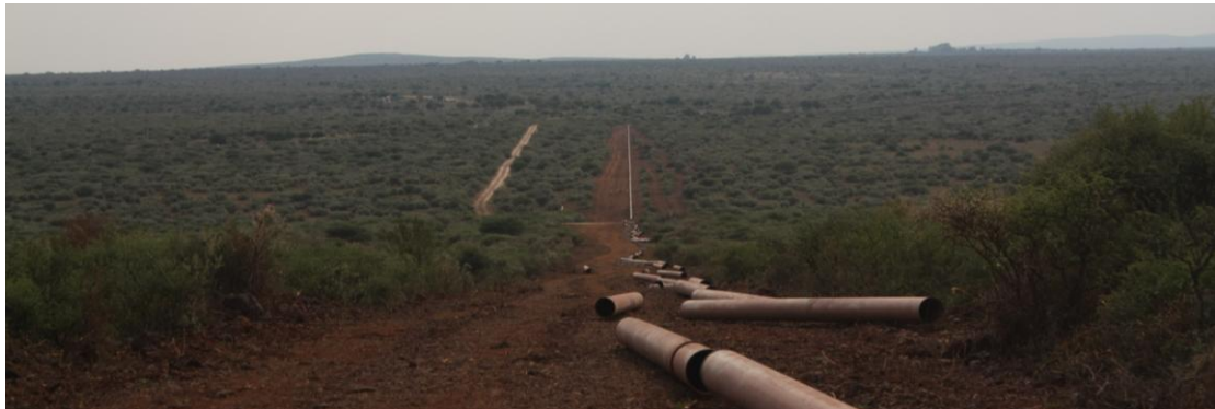
Figure 2: Pipeline in construction being installed up to the reservoir on the low hill in the north eastern portion of the site.
