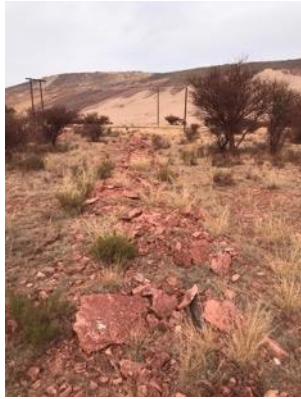
Figure 20: Sunken pipeline in the area adjacent to the proposed railway line.
