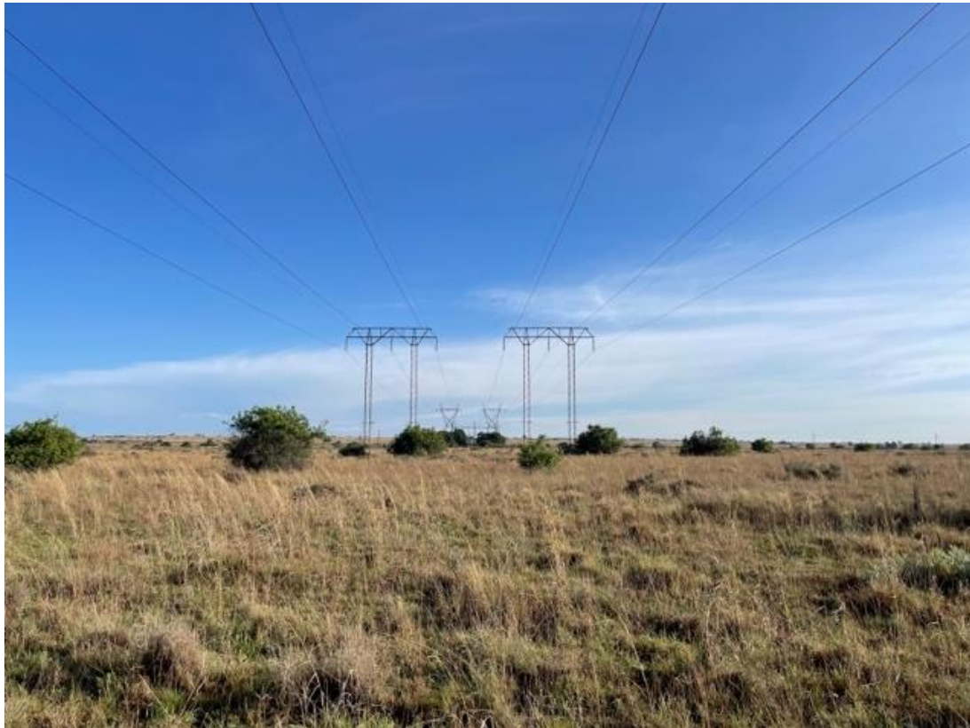
Figure 27. Presence of larger shrubs and electrical infrastructure within the proposed development footprint.
